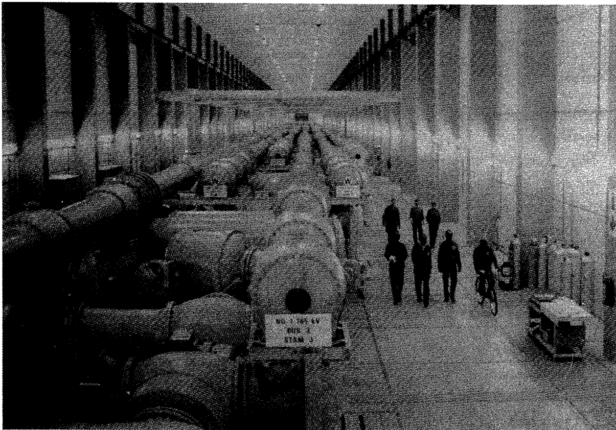
Figure 1: First 765 kV gas insulated substation ALPHA, South Africa
