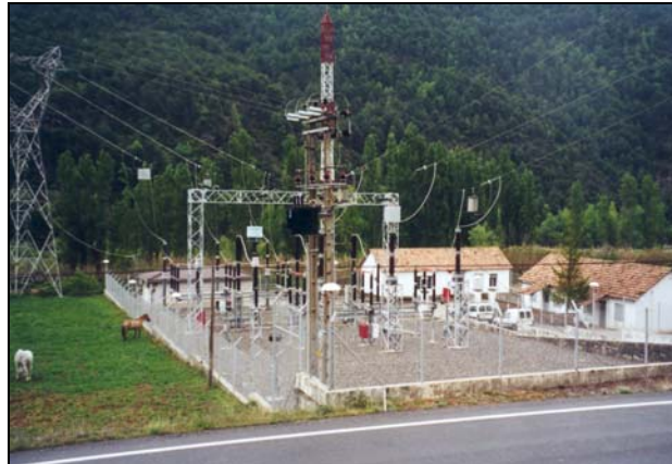
Figure 2.7: The interior of the substation is visible through the chain-link fence.
