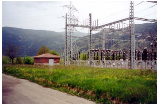
Figure 2.4: This relay shelter has been designed to reflect local architectural styles.
