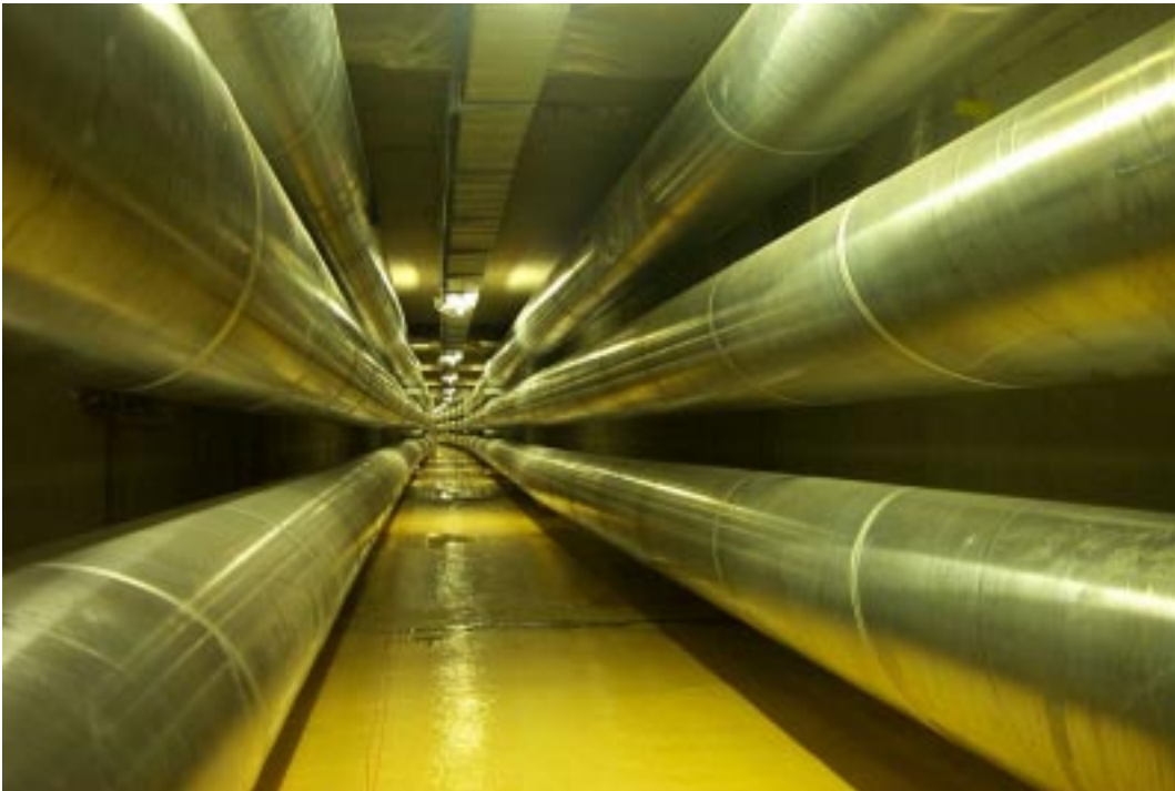
Figure 16: View of the 245 kV PALEXPO GIL.
