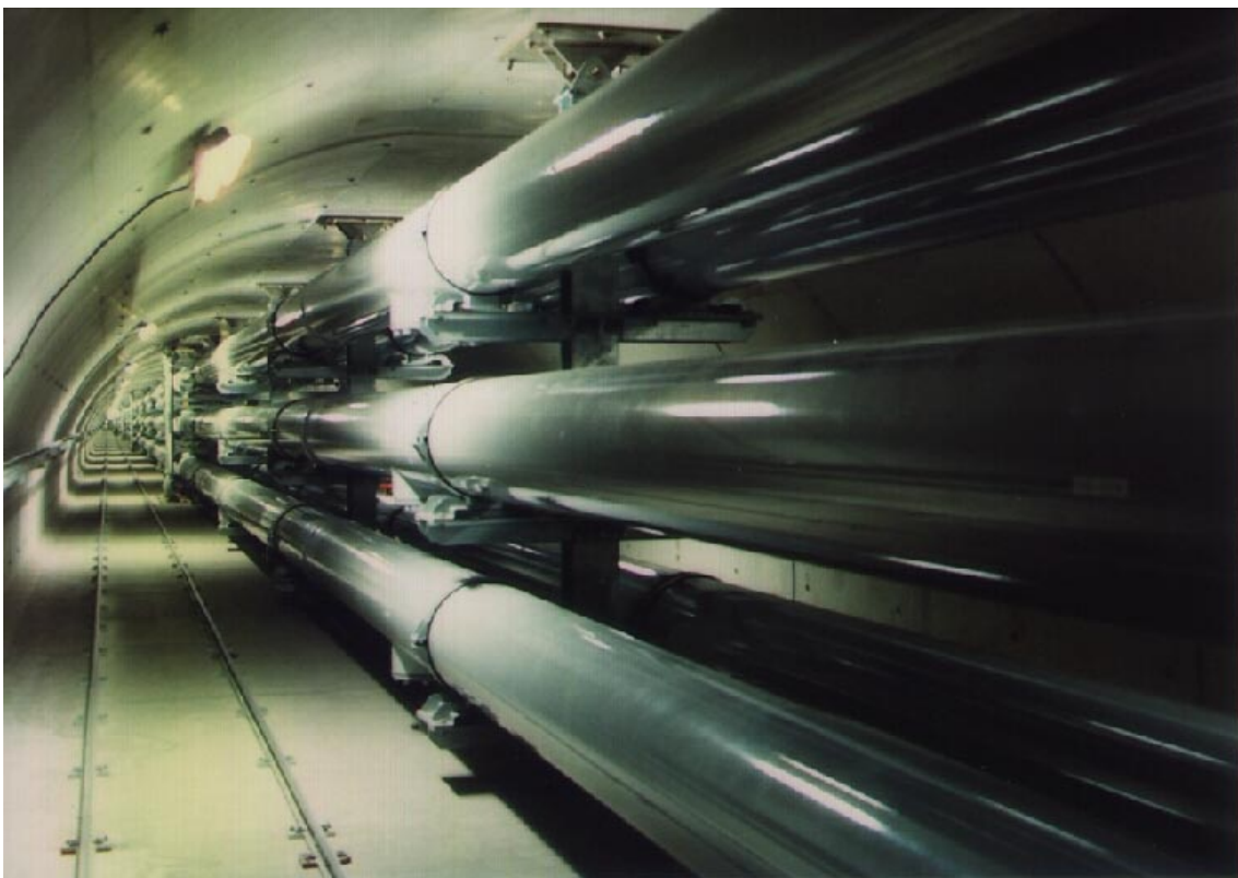
Figure 14: View of the 275 kV Shinmeika - Tokai GIL.
