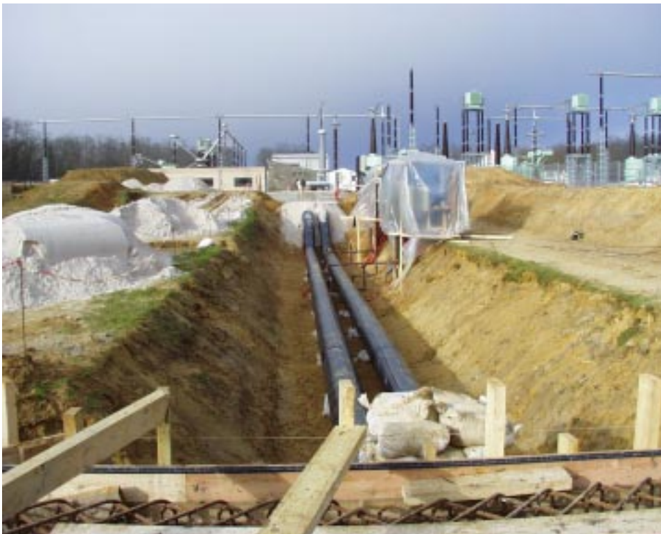
Figure 19: View of the elbows of the 300m GIL prototype and the thermally resistive backfill placed close to the GIL prototype before to bury it for the long term test.
