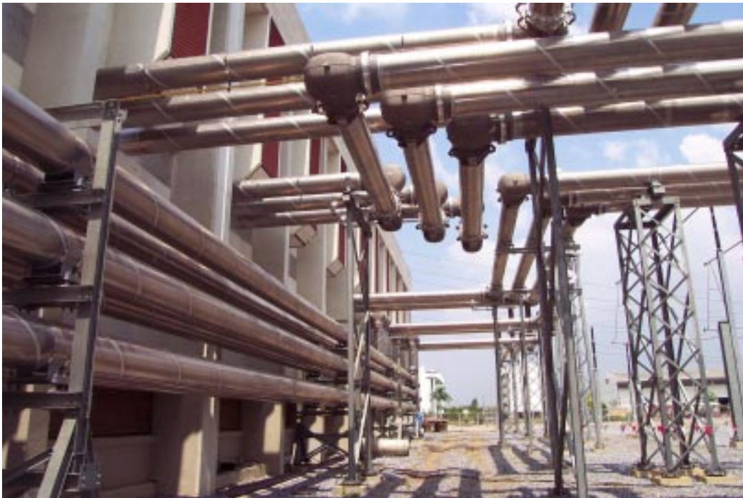
Figure 17: View of the SAI NOI 550 kV GIL.
