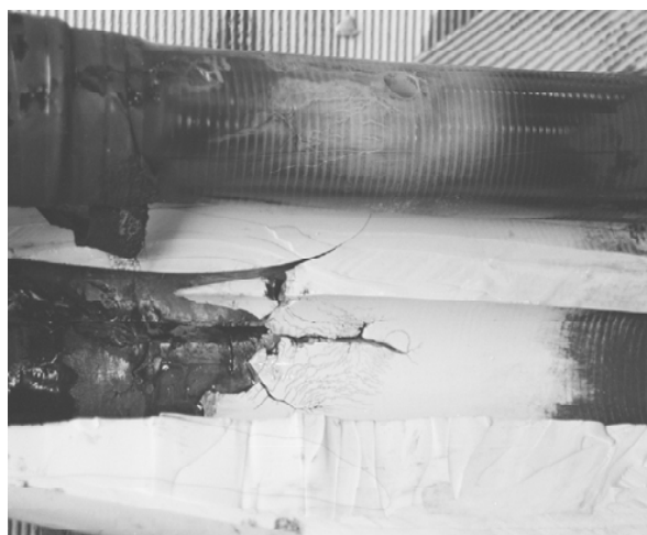
Figure 1: Electrical treeing in an interface, leading to failure of the termination [31]
