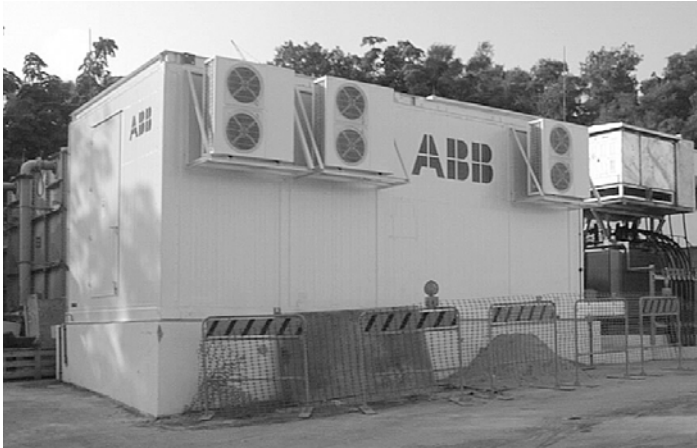
Figure 5.2.7: DVR Container with transformer in background
