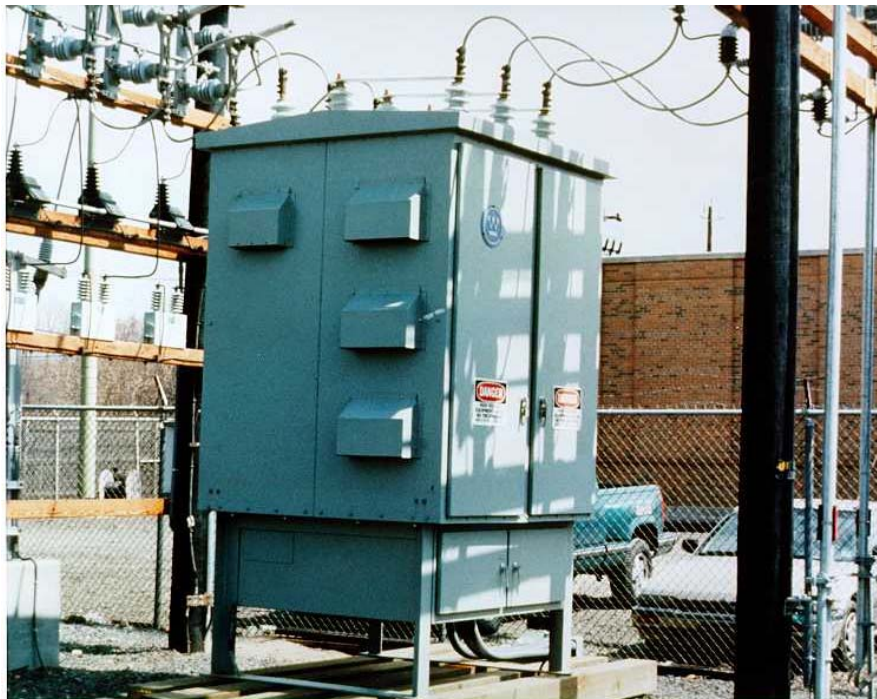
Figure 4.1.6: 13.8-kV, 600A GTO and 8-kA SCR SSB for Custom Power Applications (placed in service on PSE&G system 2/95)
