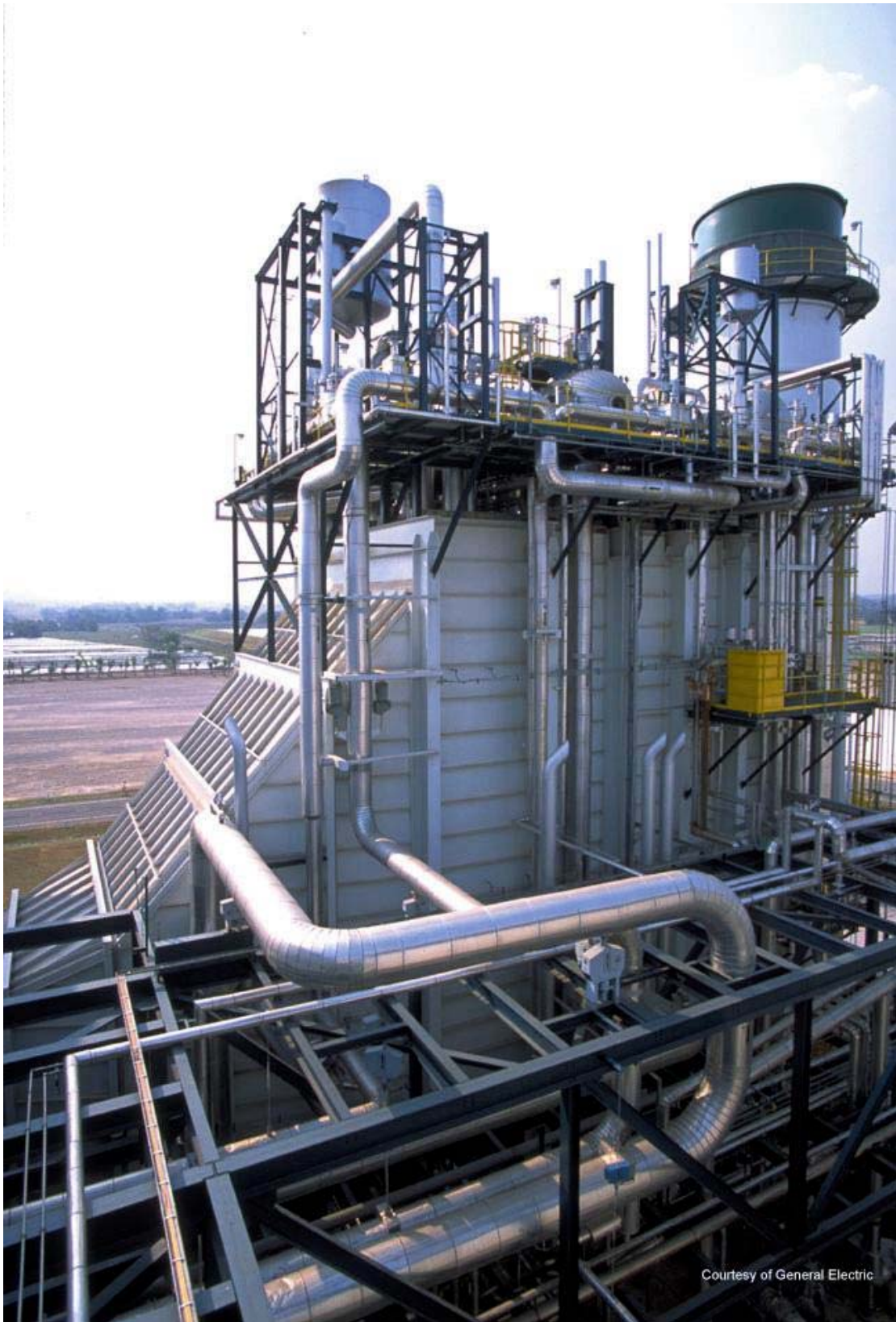
Figure 2-15: A horizontal heat-recovery steam-generator (Source: GE Power Systems)
