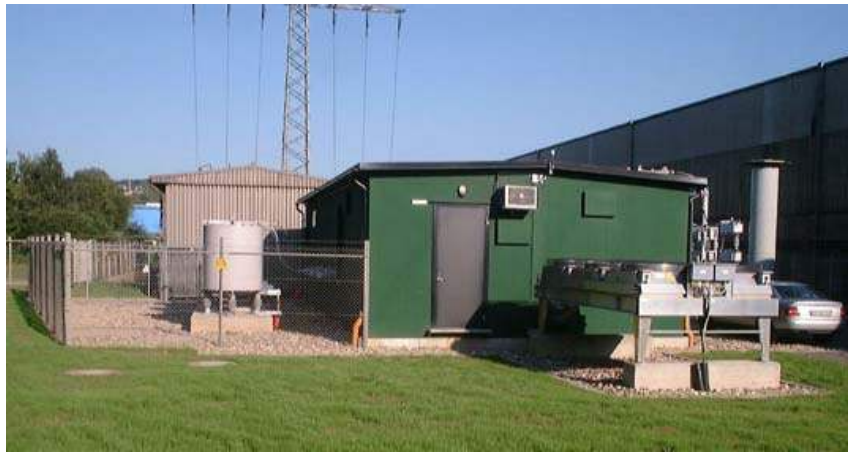
Figure 6.9 View of Trier installation showing the SVC Light equipment and the phase reactors.
