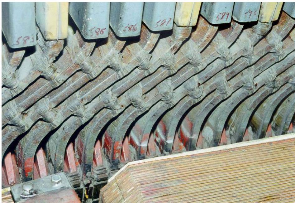
Mode 3: Endwinding discharge
