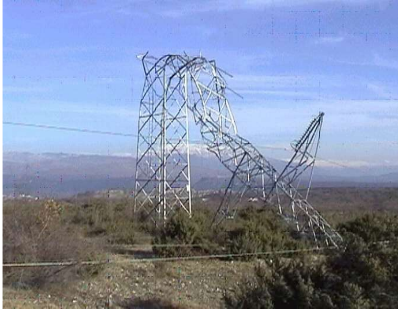
Figure 2.17 Failure of Tower during 'Bora' Wind Storm in Croatia - Jan 2003 (Photograph courtesy F Jakl)
