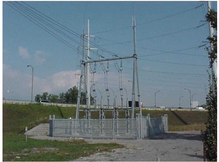
Figure 76: 120 kV Transition compound
