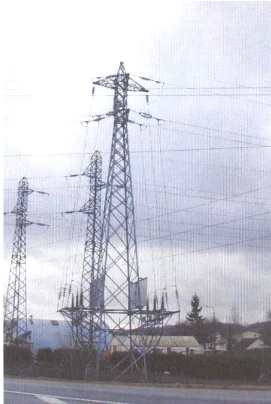
Figure 79: Transition on a lattice tower
