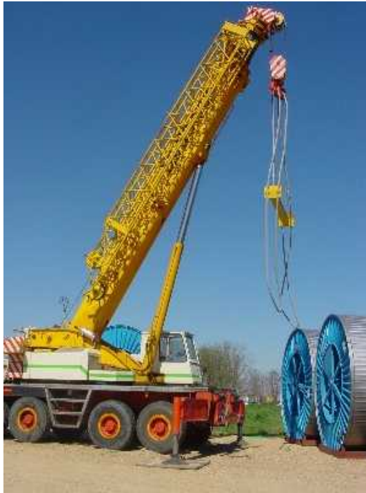
Figure 86: Crane for unloading of drums
