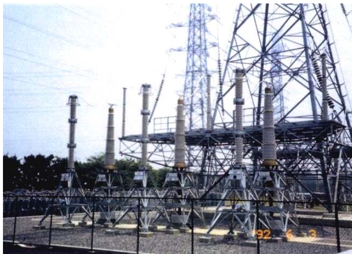
Figure 11: Example of a 275 kV transition compound (Japan)
