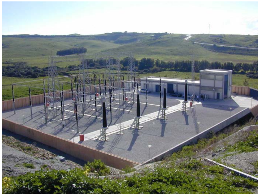
Figure 93: 400 kV Transition Compound with busbars, disconnecting switches, surge arrestors and measuring transformers
