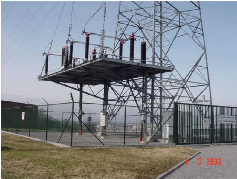
Figure 83: Transition tower with equipment on a platform
