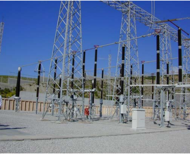
Figure 75: 400 kV transition compound
