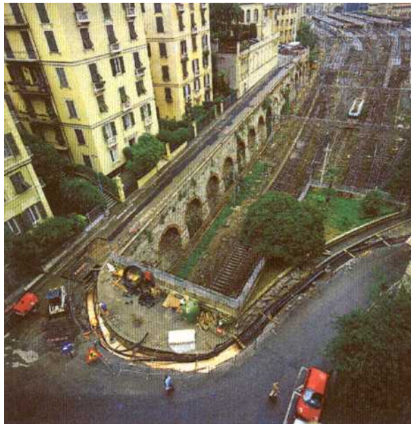
Figure 60: Example of MF shielding on 132 kV circuit crossing the city of Genoa (Italy)
