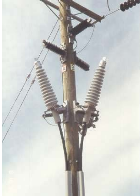
Figure 7: Transition on a pole
