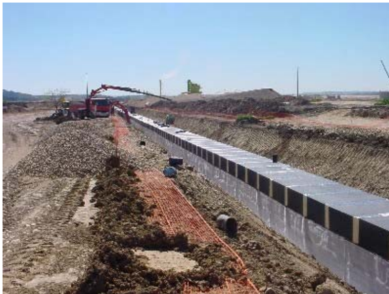
Figure 90: Civil works for the construction of a tunnel where a new 400 kV Cable system will be installed
