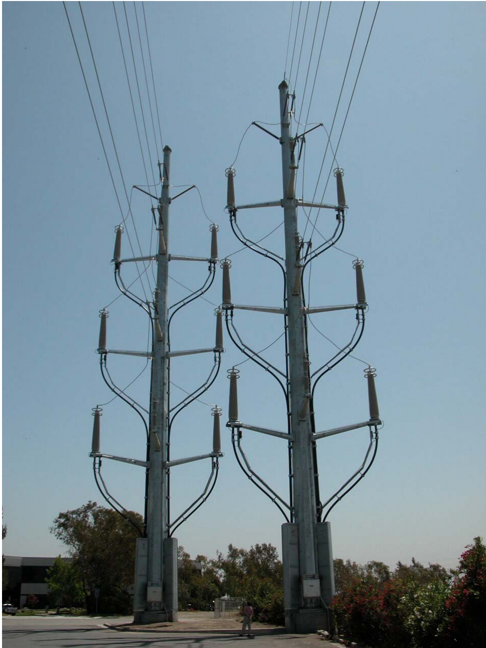
Figure 82: Transition on a pole: the cables are installed outside the pole and protected at the lower part of the structure
