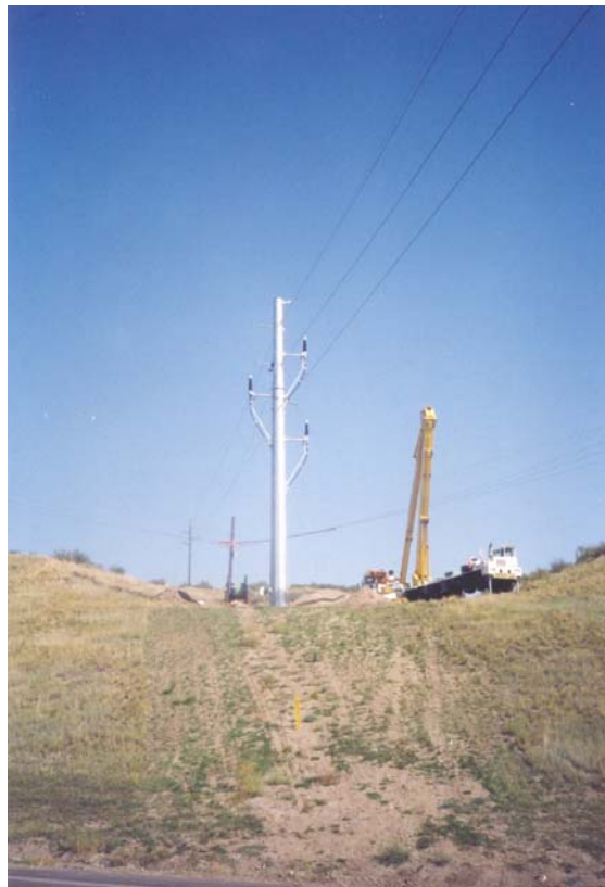
Figure 80: Transition on a pole
