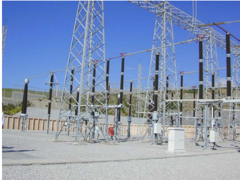
Figure 12: Equipment within a 400 kV transition compound (Spain)
