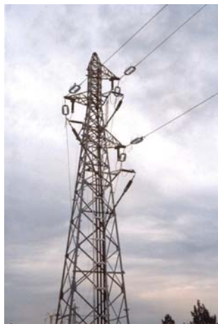
Figure 78: 100 kV Transition tower with synthetic terminations
