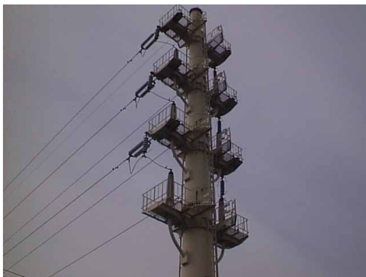
Figure 92: 66 kV Transition tower
