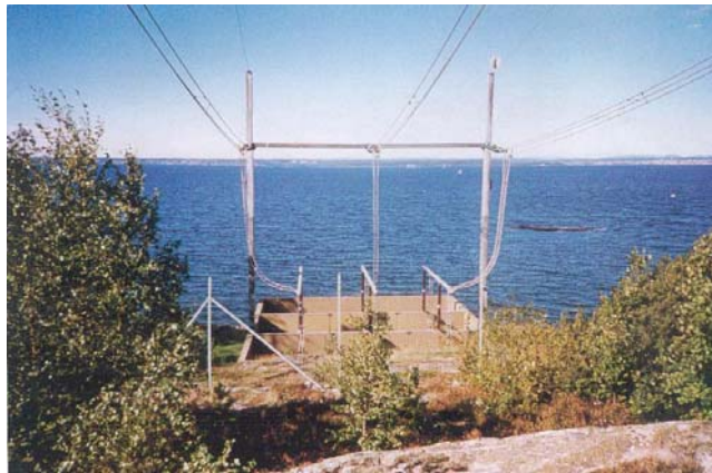
Figure 77: 400 kV transition compound surrounded by concrete walls
