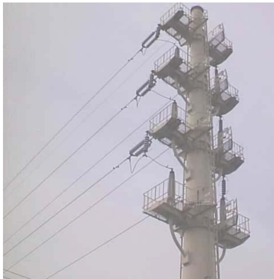
Figure 8: 66 kV terminations mounted on a tower
