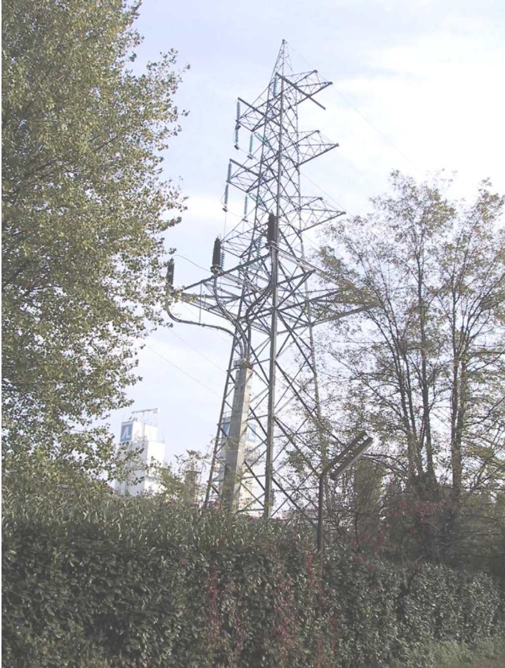
Figure 9: Terminations mounted on a platform on a tower
