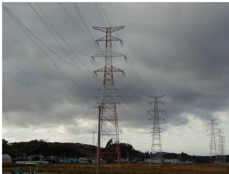
Figure 6: 4-circuit towers (275kV_66kV)
