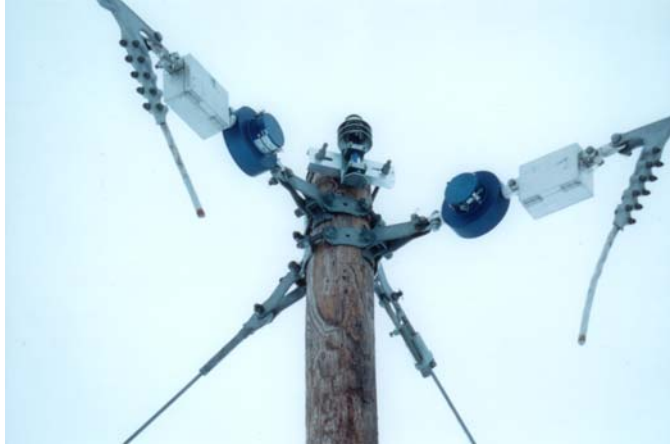
Figure 38: Top of an instrumented pole in a test span
