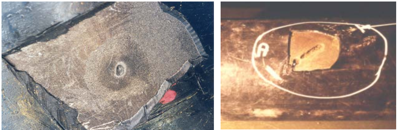
Figure 1.1: Two examples of pipeline damage caused by a.c. corrosion.
