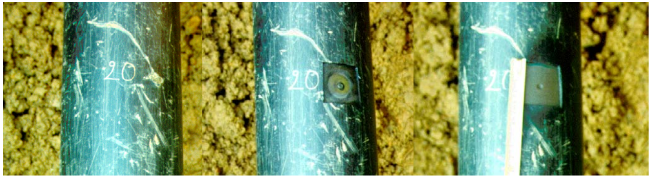
a) coating defect (15x20 mm) the hole is about a few mm 2 b) oxide (40x40 mm) and corrosion product c) pipeline corrosion (diameter = 5 mm, depth 0,5 mm)
