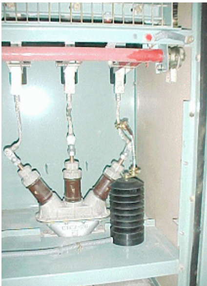
Modular cubicle with tripolar cable
