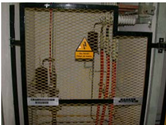
Masonry compartment with XPLE unipolar cables
