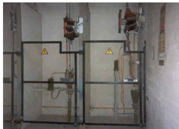
Masonry compartments with tripolar cables
