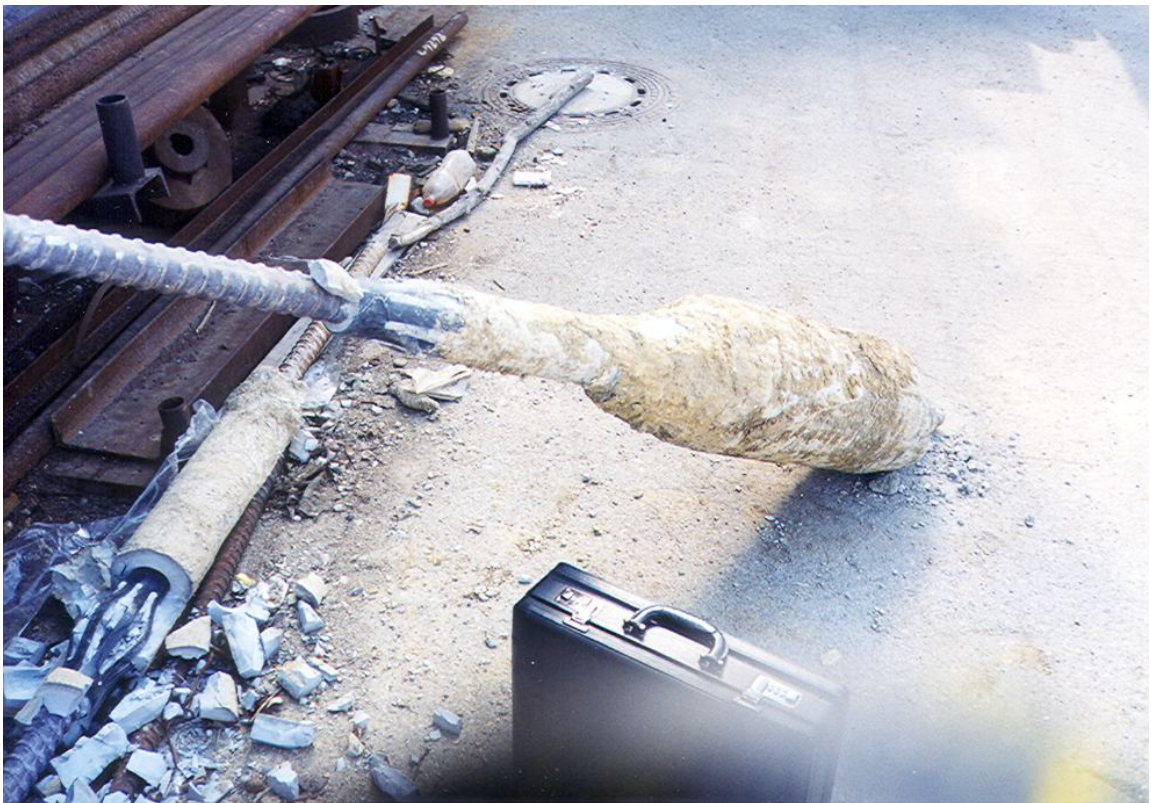
SLOVENIA, Cylindrical extension of the lower part of the micropile; used in hard expanding clay
