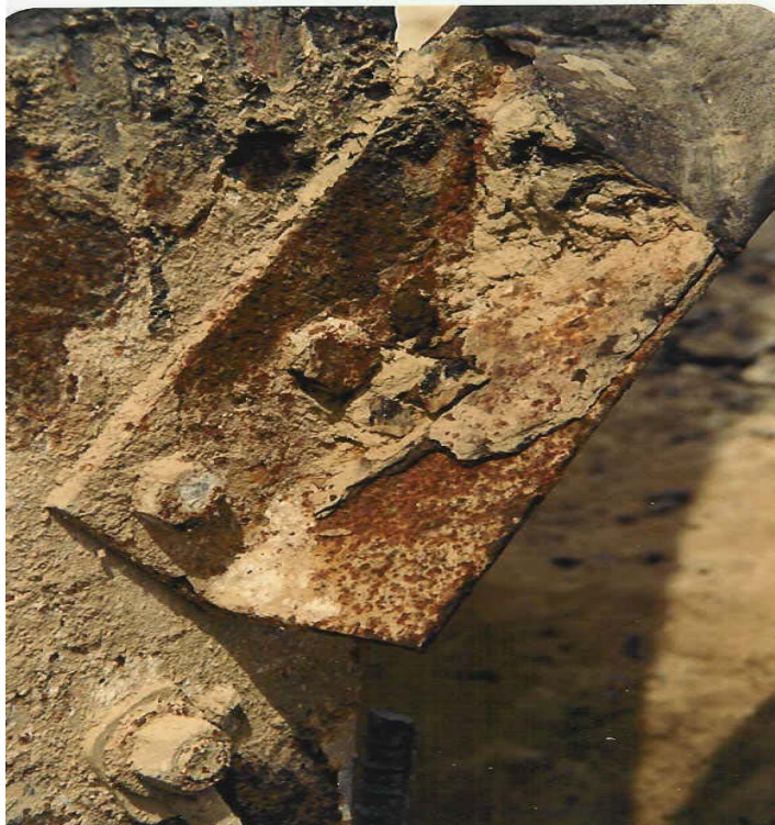
Figure 2.8B – Corrosion of tower bracing member after removal of the muff concrete.
