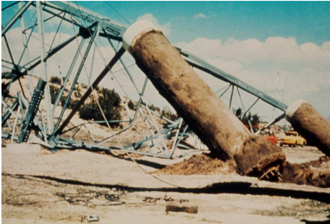
Figure 1.3 – Failure of a 500 kV Suspension Tower Drilled Shaft Foundation
