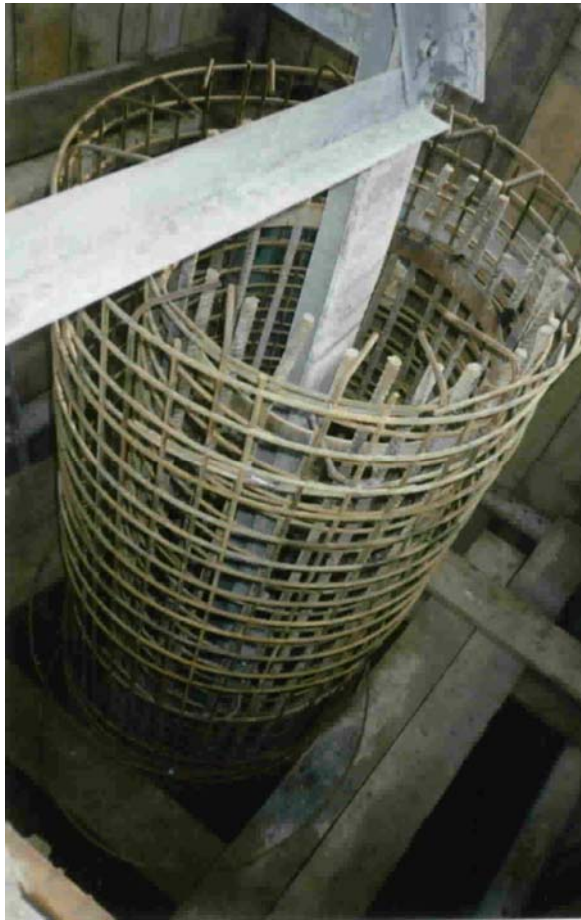
Figure 3A.11a – Bored pile 1.3 m diameter single pile per leg 380 kV lattice steel tower
