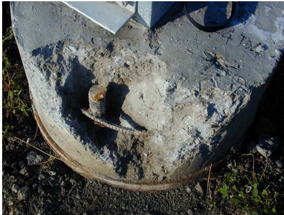
Figure 2.4 – Drilled shaft foundations failure to adequately remove all of excavation material during concrete placing (Key 7 & 10)
