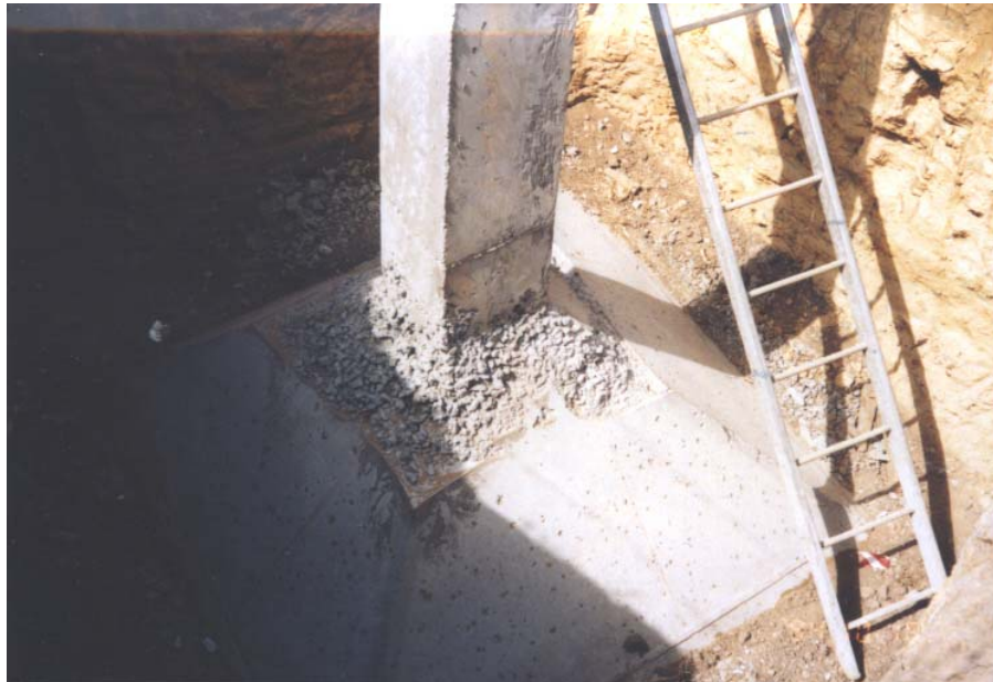
Figure 2.2 – Separate foundations poor compaction of concrete at the chimney – pyramid joint (Key 8)
