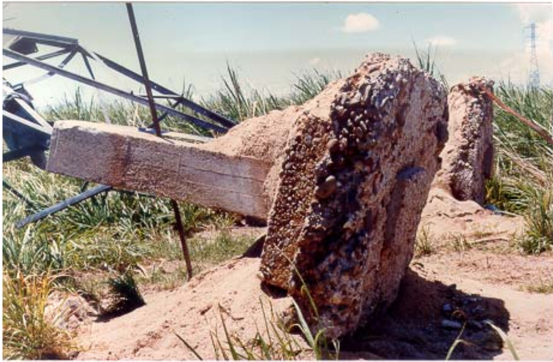
Figure 8.1 ~ Failure of the Tully Falls – Townsville 132 kV OHL, Queensland, Australia
