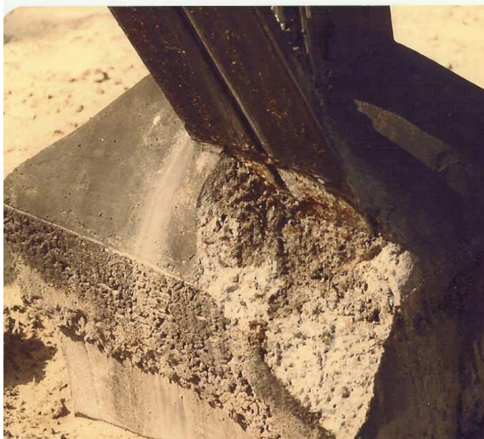
Figure 2.8A – Corrosion of stub & tower bracing member
