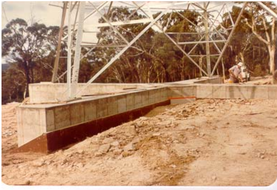
Figure 3A.12 – Details of cruciform foundation for 330 kV lattice steel tower located in Hunter Valley coalfield, N.S.W. Australia
