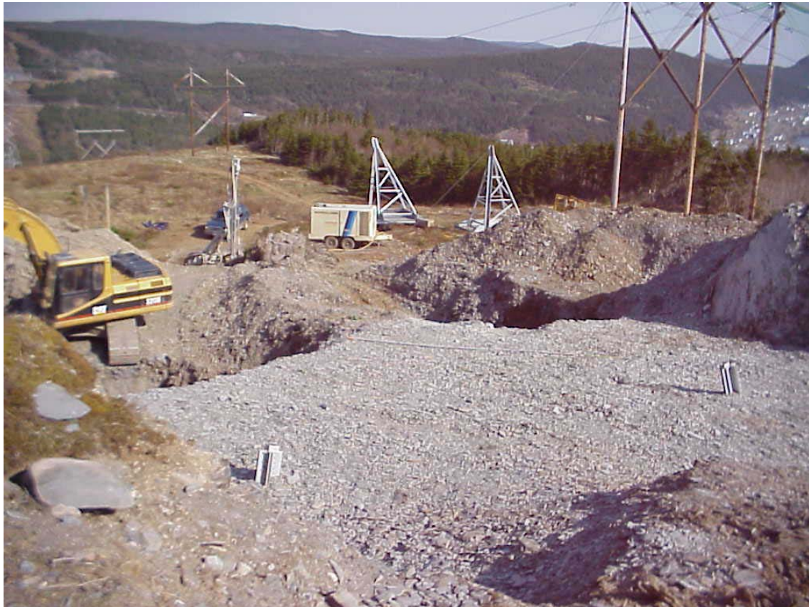
Figure 3A.9c – Completion of the backfilling for the nearest tower legs and excavation for the far two legs.
