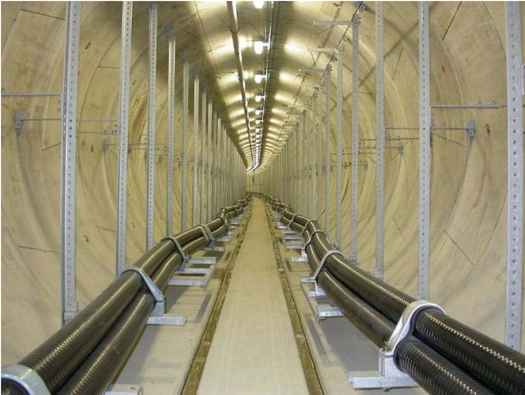
345 kV Cables installed in a long Tunnel in Korea
