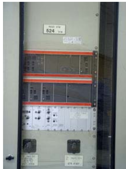
Figure A3-4: New Digital Transformer Protection Panel
