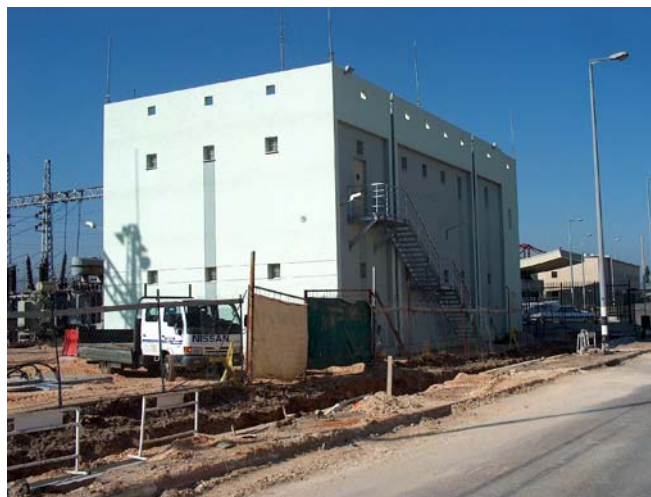
Figure A4-6: New Control & MV Building
