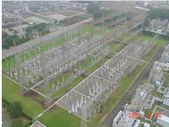
Figure A6-1: The Original 275 kV Substation Comprising Double Deck Bus Configuration
