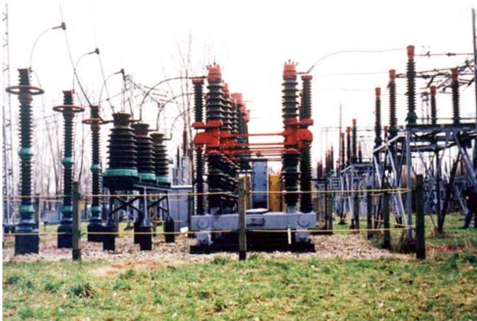
Figure A2-2: Part of Warszawa-Batory Substation before Modernization
