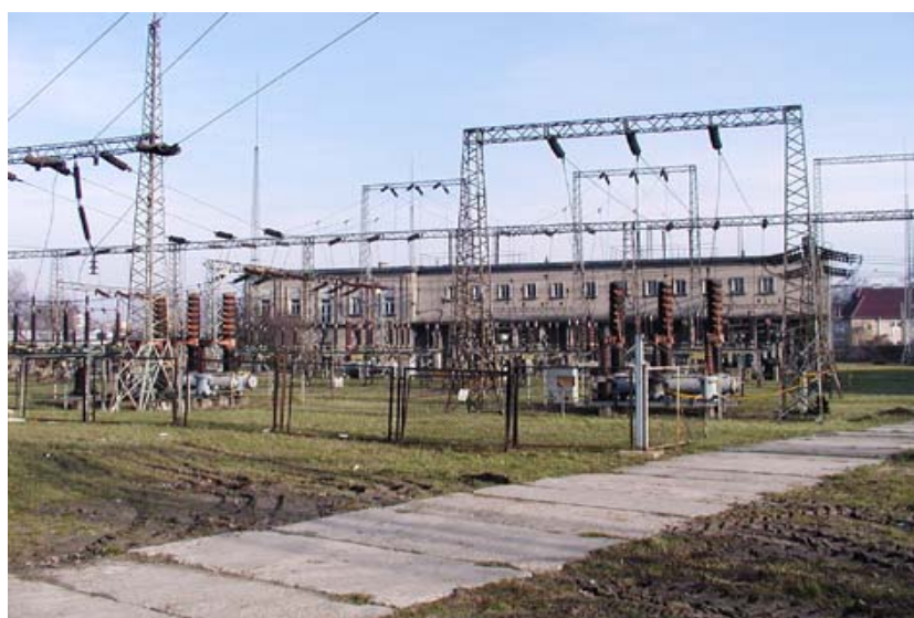
Figure A2-5: Part of Warszawa-Zachodnia Substation before Modernization.
