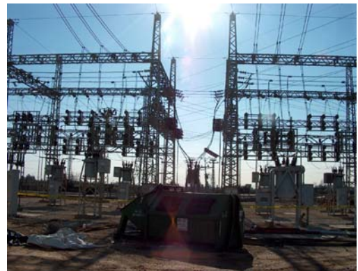
Figure A4-5: Old MV Switchgear
