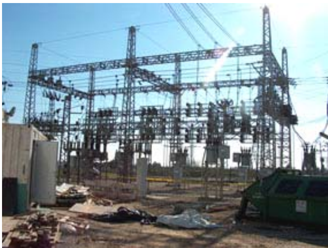
Figure A3-1: Old Outdoor Bulk Oil MV Switchgear
