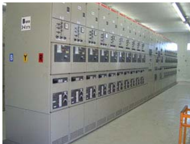
Figure A3-2: New Indoor SF 6 MV Switchgear
