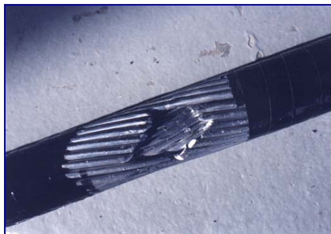
Figure 8.52: Damaged conductor under the metal-to-metal clamp in the 450-m span at the end of the second test
