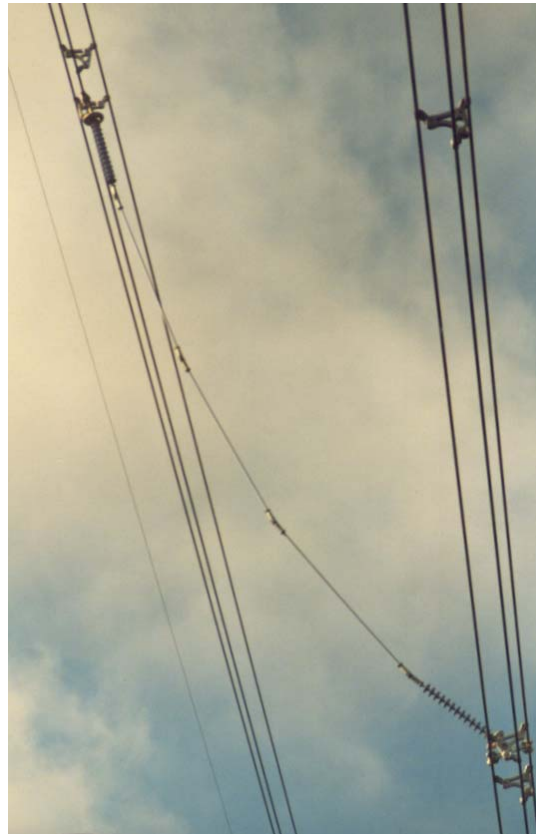
Figure 8.6: Flexible polymeric interphase spacer installed on a triple bundle 500 kV line in Manitoba Hydro [Pon and Havard, 1994]
