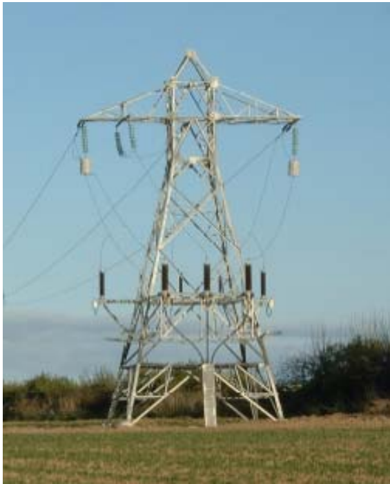
Figure 3.17 Terminations mounted on a platform on a 110 kV overhead line tower
