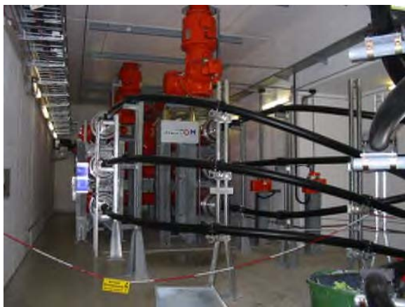
GIS terminations in the transition area
