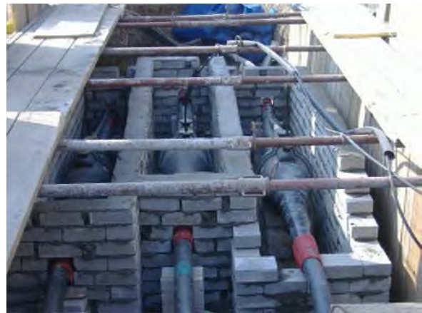
Figure 2: 380 kV cable joint bay
