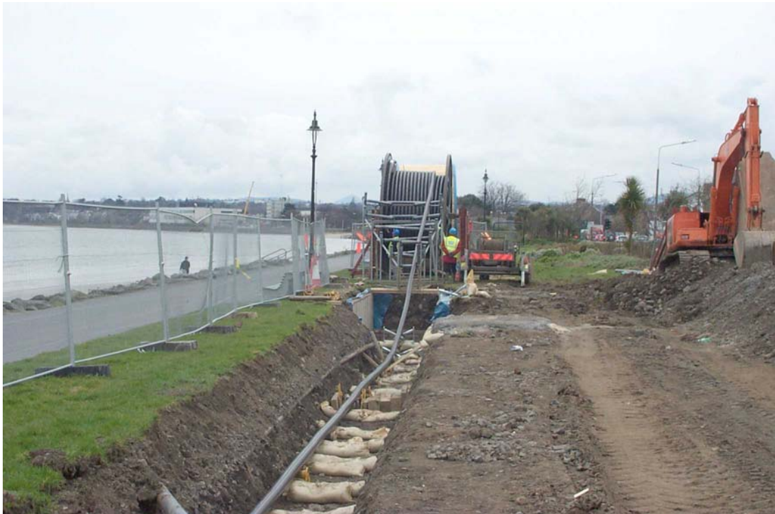
Figure 3.11: Cable trench on open land
