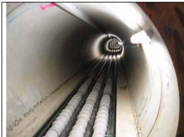
Fig. 4: Picture of the tunnel laying with cable protected by covers (removed after completion)
