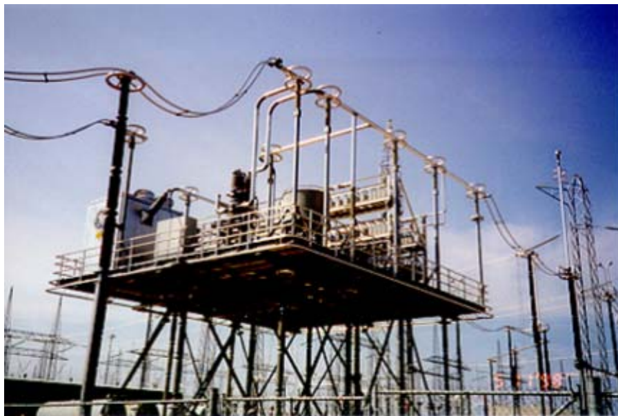
Fig 3: example of 735 kV capacitor bank
