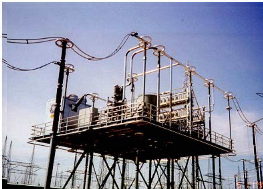
Fig. 3 Example of a 735 kV Series Capacitor Bank
