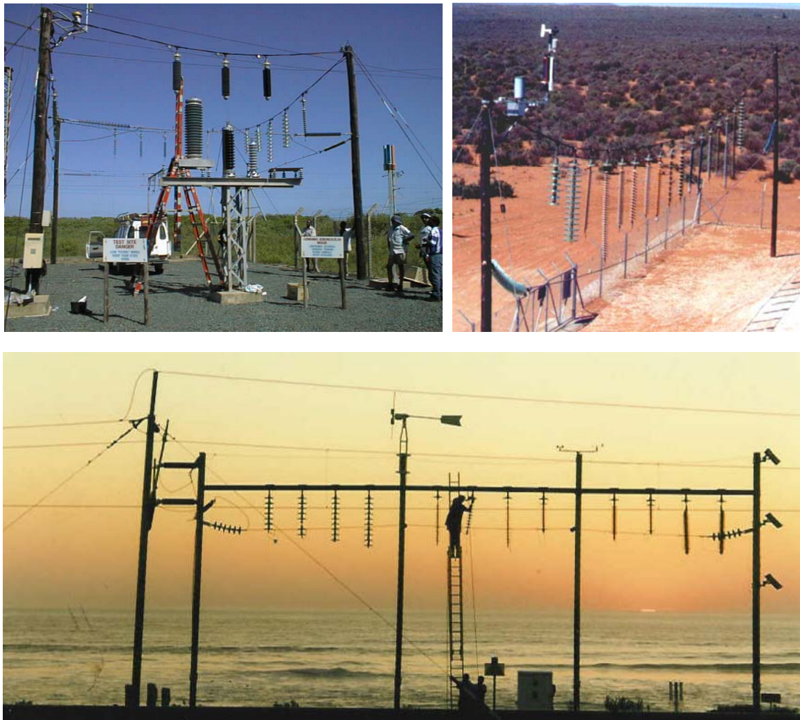
Figure 2. On-line insulator test stations.
