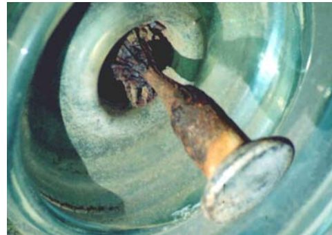
(n) Pin corrosion
