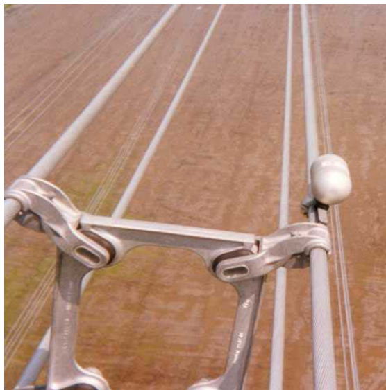
Figure 18: Vibration recorder Pavica installed near a spacer damper clamp.
