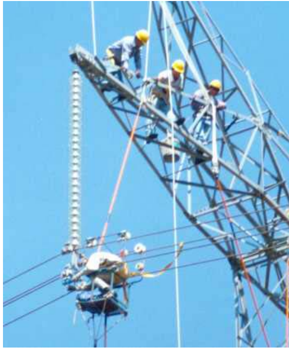
Figure 20: Installation of a vibration recorder on an energized line using the bare hand technique.
