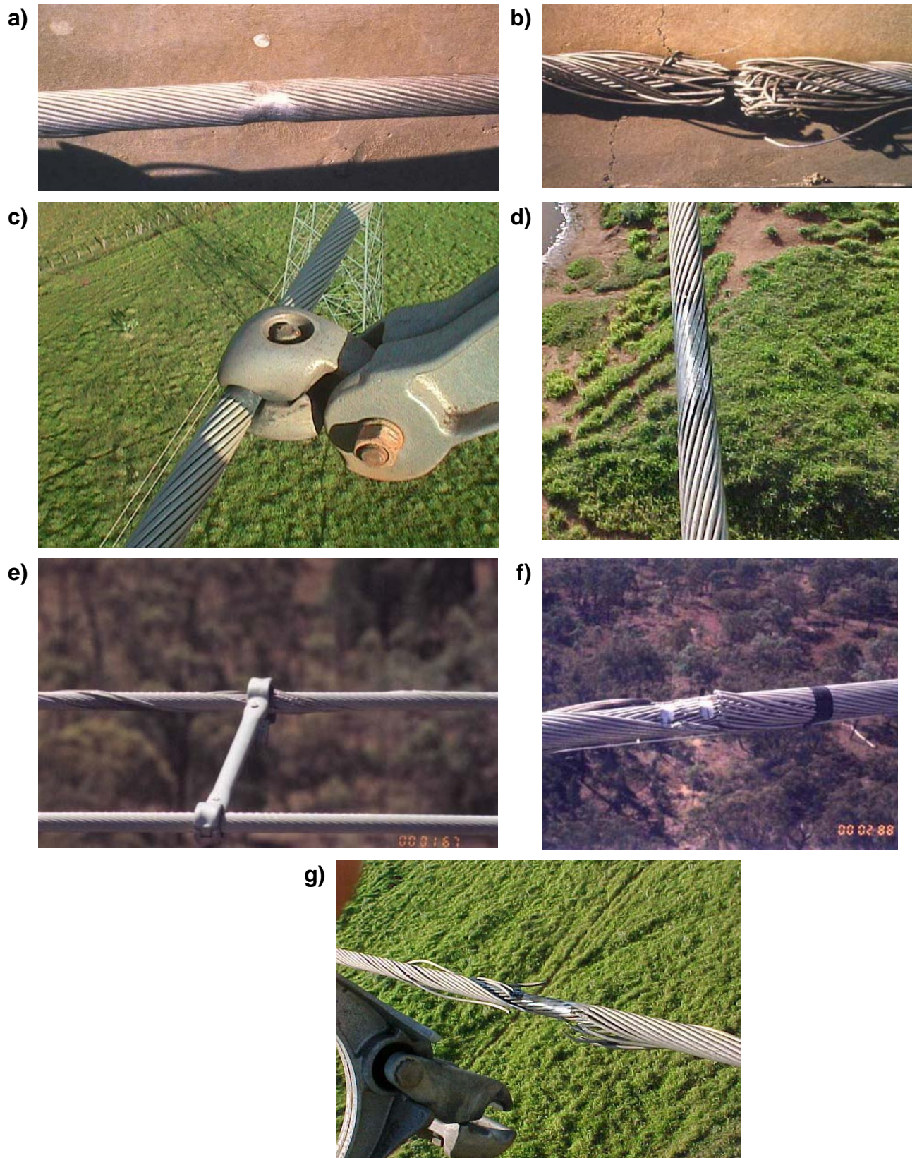
Figure 15: Wear and failure of conductor strands due to spacer clamp loosening.
