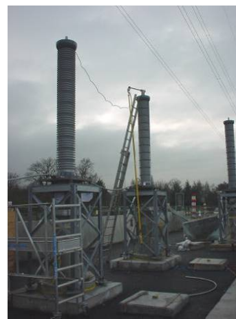
Figure 71: On site HV testing Connecting to the bushing
