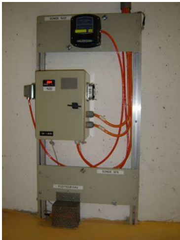
Figure 57: Monitoring the air quality by measuring oxygen and SF 6 including a water sensor in the tunnel for safety
