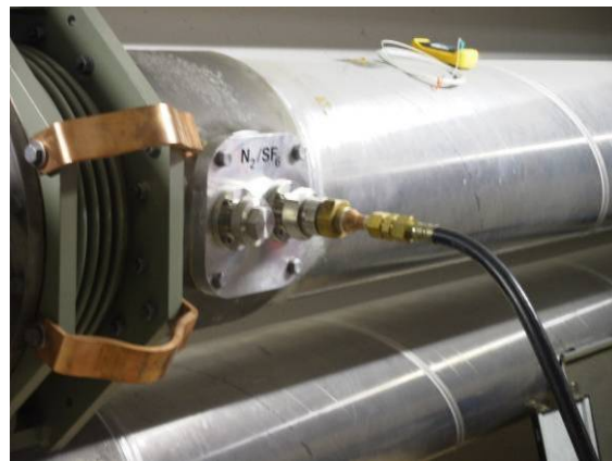
Figure 68: Gas filling Dilo valve to connect gas handling device
