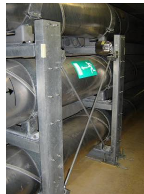
Figure 56: Structure for fix point of the GIL in the tunnel
