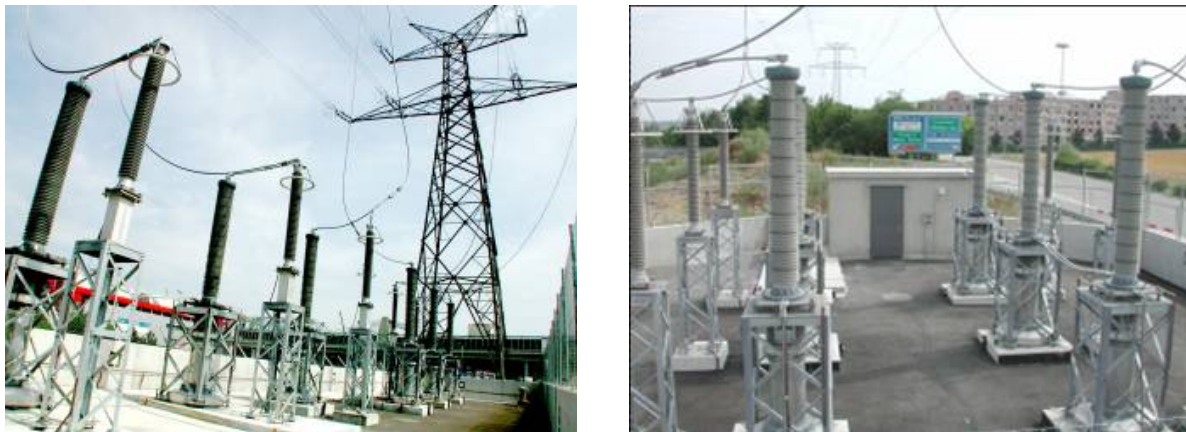
Figure 42: GIL termination, transition to overhead line.
