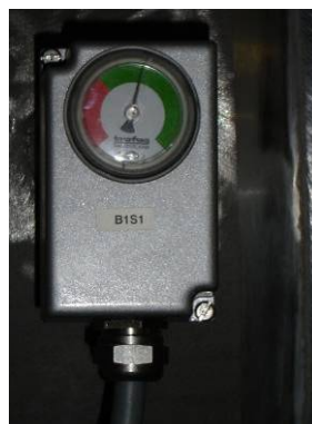
Figure 50: Density meter for gas mixture monitoring
