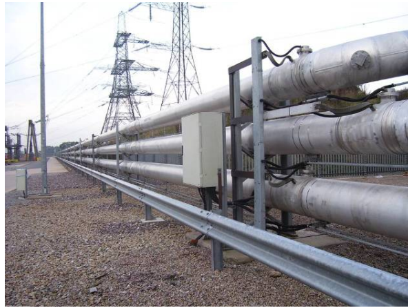
Figure 15: Above ground installation inside the substation
