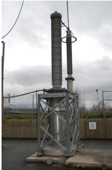
Fig. 53: Connection to overhead line by bushing with parallel surge arrester
