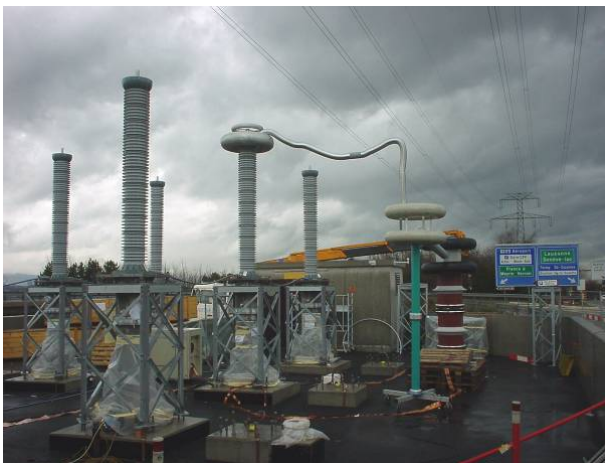
Figure 70: On site HV testing Air insulated high voltage resonance test set-up
