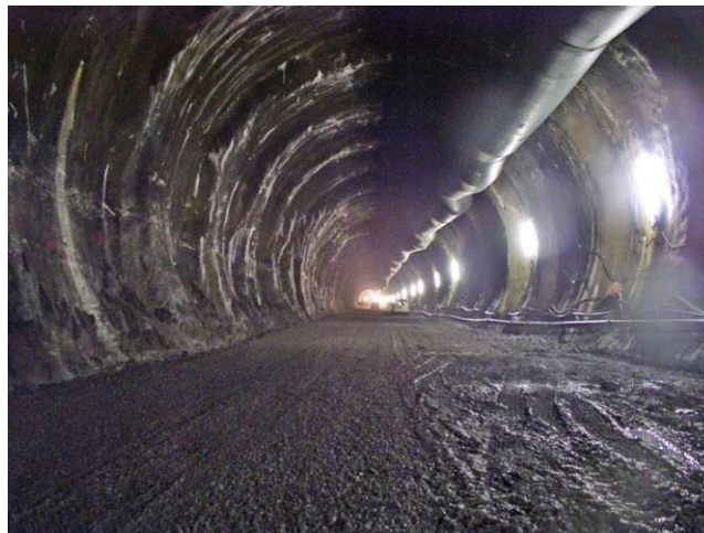
Figure 28: Railroad tunnel of Unterinntaltrasse Brixlegg Tirol, Austria, a double track railroad tunnel
