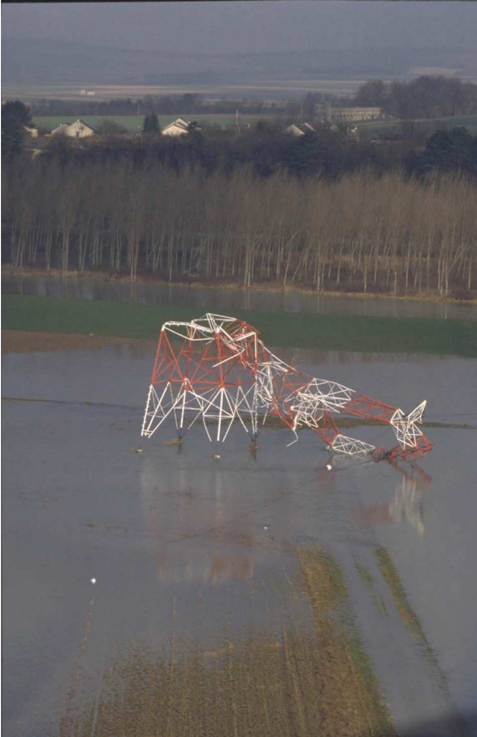
Figure 3 - December 1999 windstorm in France (RTE)
