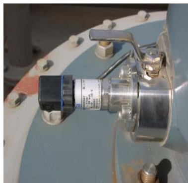
Figure 4 Bushing pressure sensor
