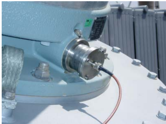
Figure 2 Example of a bushing tap voltage sensor
