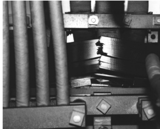
Figure 4: Collapse of winding end support.
