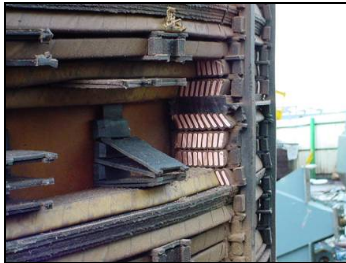
Figure 8: Conductor tilting (normally, all conductors should be completely vertical).
