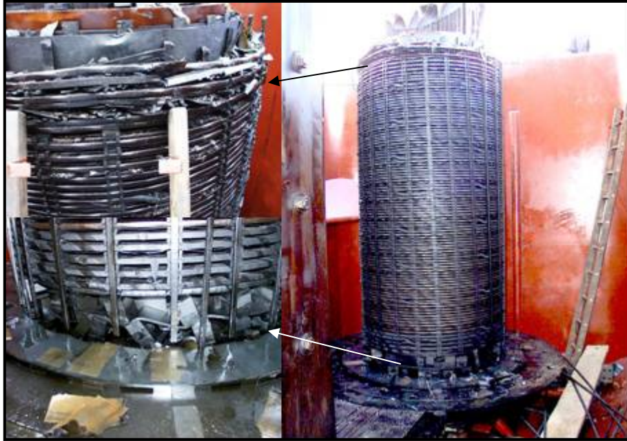
Figure 6: Axial collapse after clamping failure.
