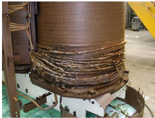
Figure 36: Localized winding displacement on the regulating winding caused by a tap changer fault.
