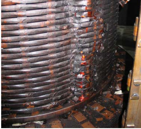
Figure 1: Radial buckling of inner winding.
