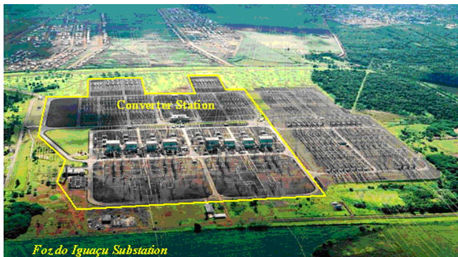
Fig.2.5.2 Foz do Iguaçu substation contains both the HVAC switchyard for three 800kV circuits and the HVDC converter substation equipment/switchyard (HVDC link rectifier side)
