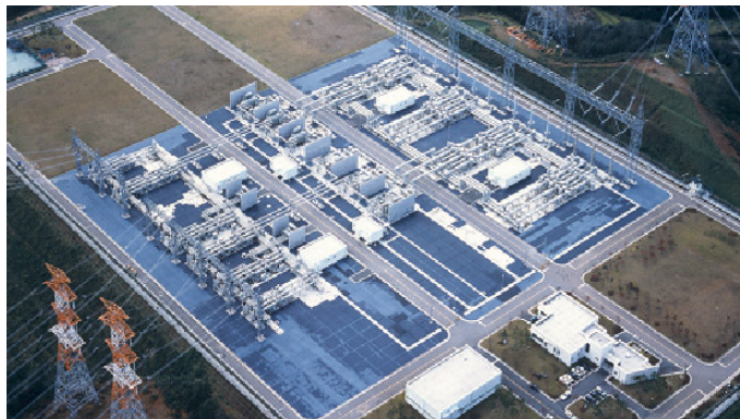
Fig.2.4.2 KEPCO 800 kV GIS substation
