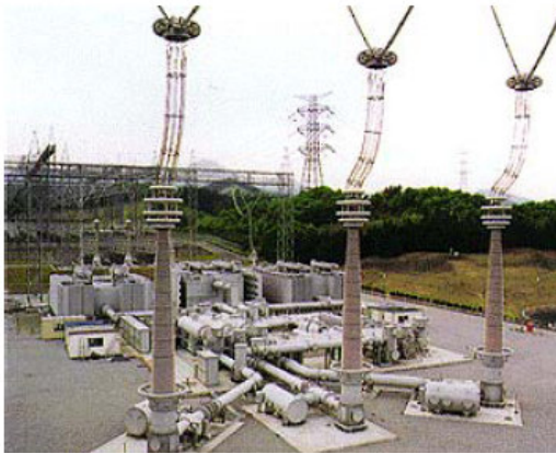
Fig. 2.9.6 TEPCO testing station
