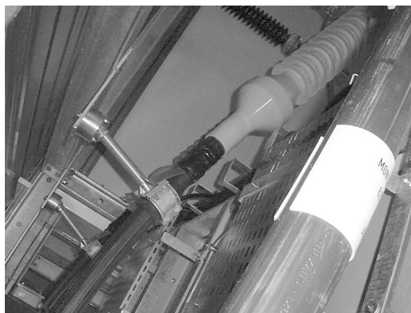
Short HV terminations installed in an indoor substation.
