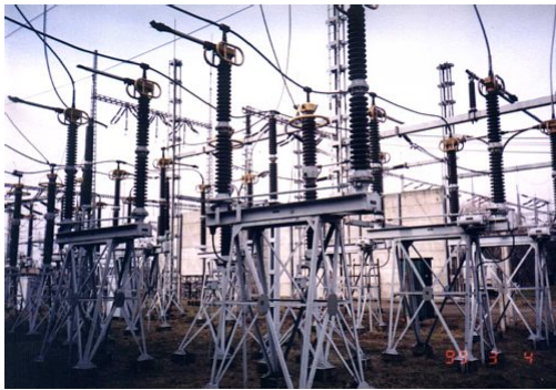
Photo 1: Old 220 kV switchgear
