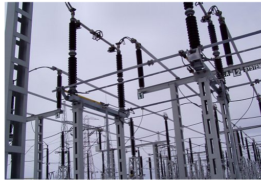
Photo 2: New 220 kV switchgear
