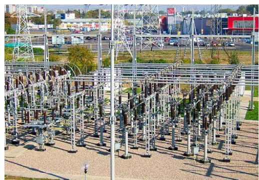
Photo 4: New 220 kV switchgear
