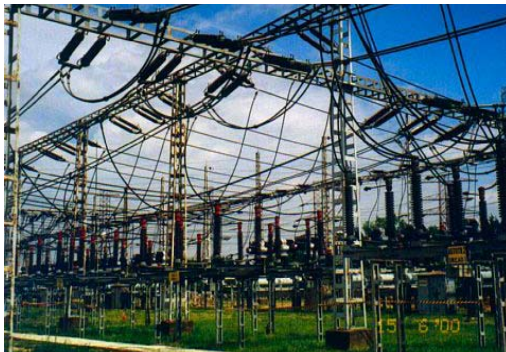
Photo 3: Old 220 kV switchgear
