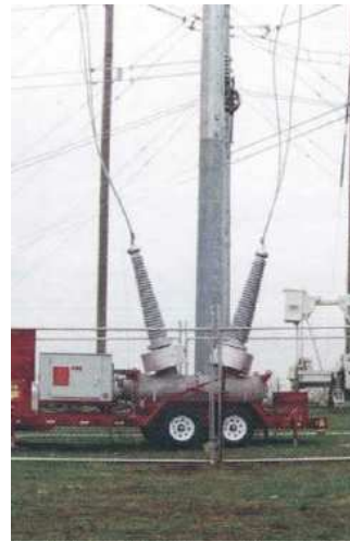
Mobile 345kV Breaker.
