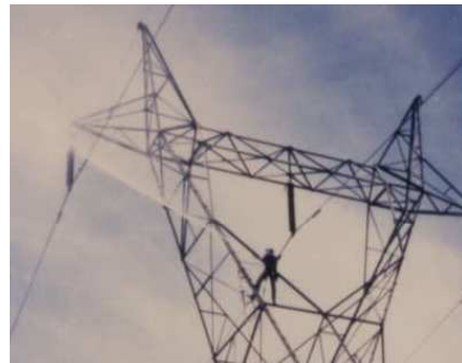
Above, typical insulator washing on +/- 500kV DC and 230kV lines
