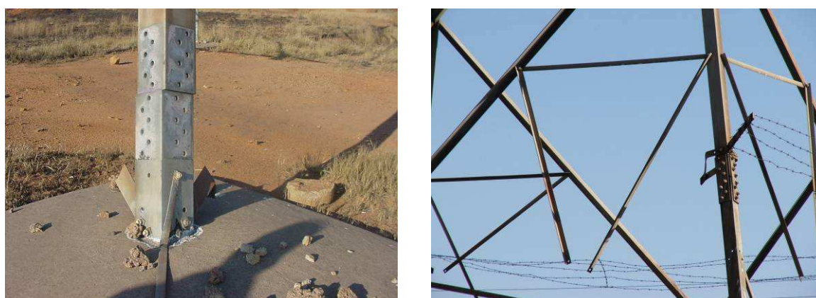
Figure 6-2: Theft of steel parts
