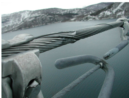
Figure 6-13: Wear and Broken Wires Due to a Loose Damper
