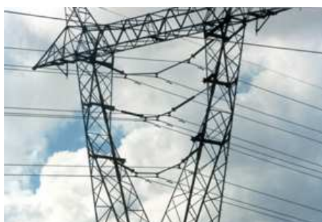
Figure 4-10: 230 kV Experimental HSILL Transmission Line
