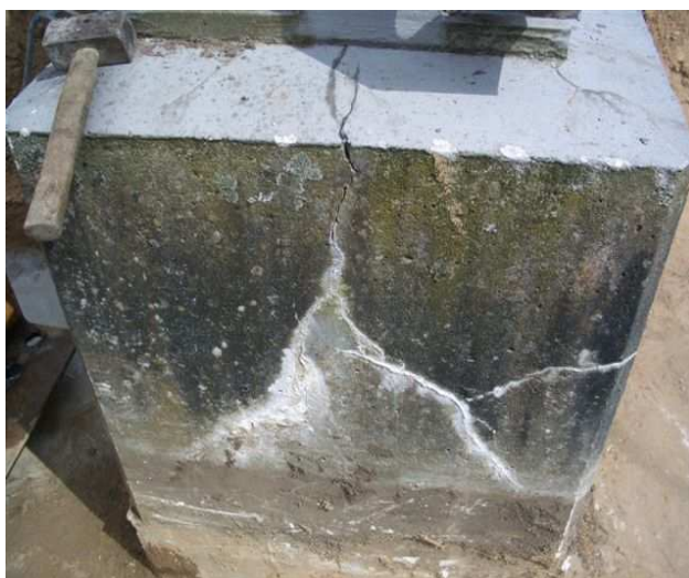
Figure 6-3: Cracking of concrete foundation
