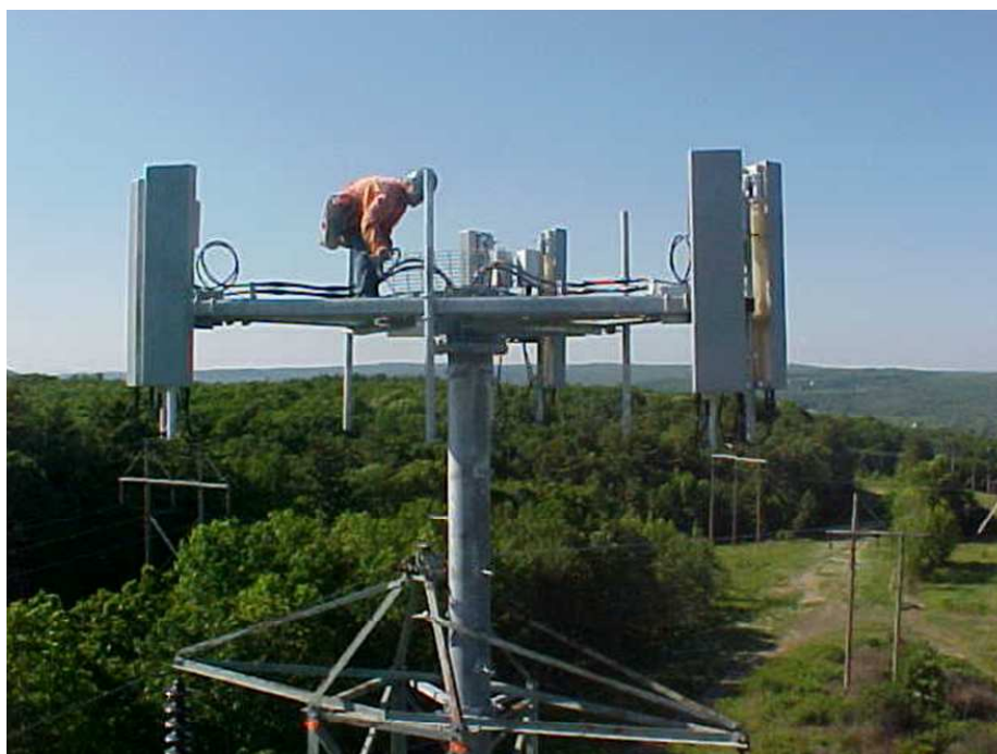
Figure 7-2: Worker on pipe extension to a double circuit 115 kV lattice steel tower with antenna mount platform
