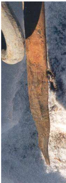
Failed anchor rod (5m below ground)
