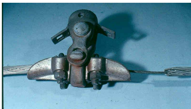
Figure 6-12: Fatigue has Lead to Broken Wires in a Supporting Clamp Due to Vibration
