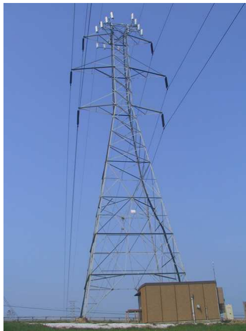
Figure 7-1: Direct mount of telecommunications antenna to a double circuit 230 kV lattice tower between shield wire and top conductor arm. Note location of communication control building and coax cable installed on cable ladder.
