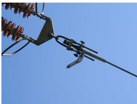
Figure 6-14: A Swinging Jumper has Lead to a Broken Conductor Adjacent to a Dead End Tension Joint
