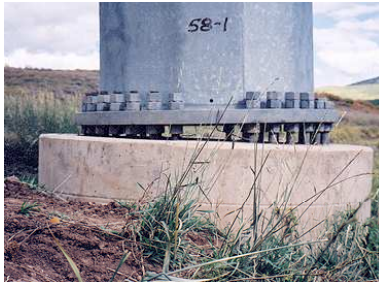
Figure 1: A close up of Structure showing how much the anchor bolts have been adjusted to compensate for the shifting ground due to landslide
