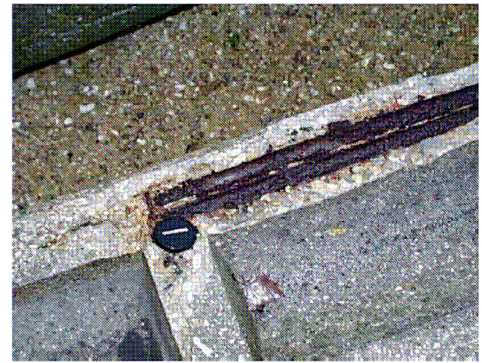
Typical pathology on concrete poles : outer part of concrete damaged as a consequence of a corrosion process on steel reinforcing bars
