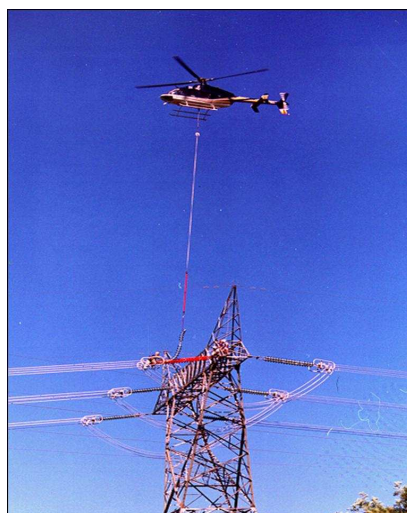
Figure 6-10: Replacing Faulty Insulator in a Dead-End Insulator String, Live Line Maintenance is Used
