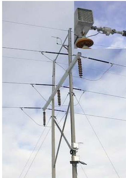
Figure 4-7: Conductor Tension Monitor
