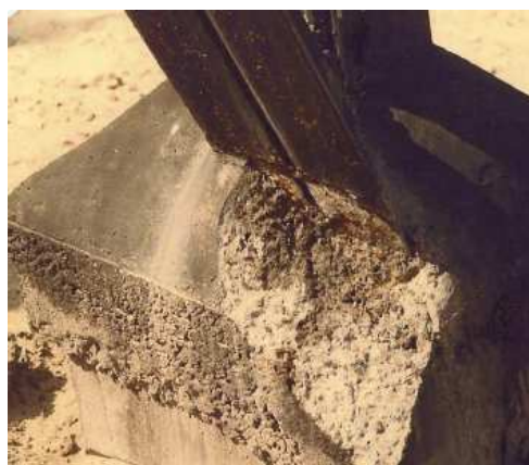
Figure 6-4: Corrosion of Stub and Tower Bracing Member
