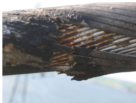
Figure 6-11: Broken Wires Due to Corrosion and Corrosion Fatigue Beneath a Damper
