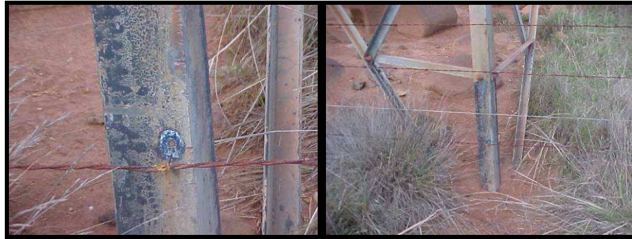
Figure 5-10: Typical Evidence of Structure Potential Rise and Flashover to Adjacent Metallic Fence
