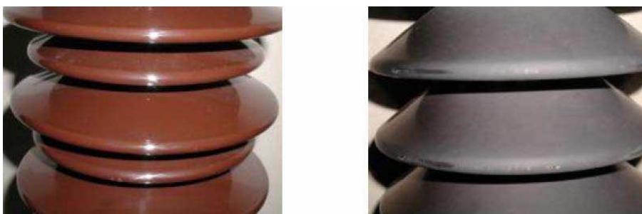
Figure 6-8: A new ceramic insulator on the left and a ceramic insulator after 30 years in operation on the right – glazing of the surface is damaged, the surface is rough and different kinds of fungi contribute to it's deterioration. Consequently leakage distance of such insulator has decreased due to increased conductivity of the surface and a number of flashovers have occurred.
