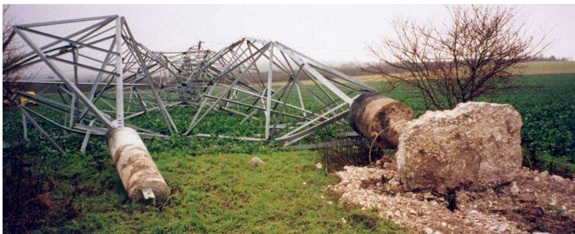
Figure 5-1: Foundation Failure after Windstorm
