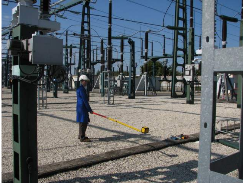
Figure 6 : electric field measurement using a hand-held stick (photograph RTE)
