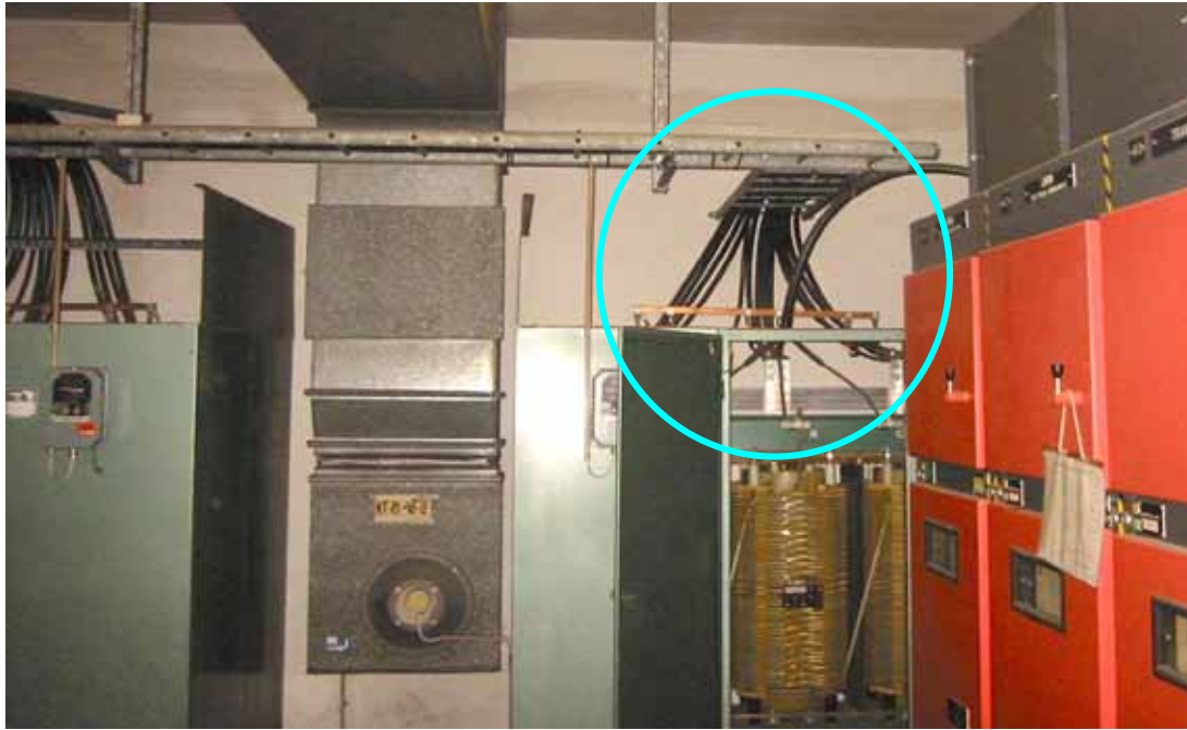
Figure 3.3.1 Identification of a part of the power system as the main source of magnetic fields; experiments with this section were performed in the lab which lead to an effective mitigation design.
