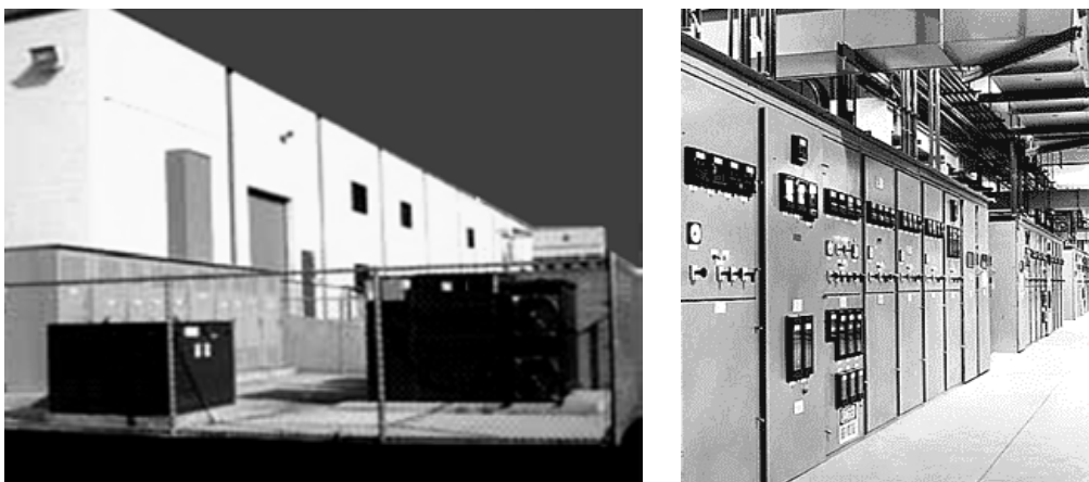
Figure 5.4.15 Two types of substations in an industrial environment.
