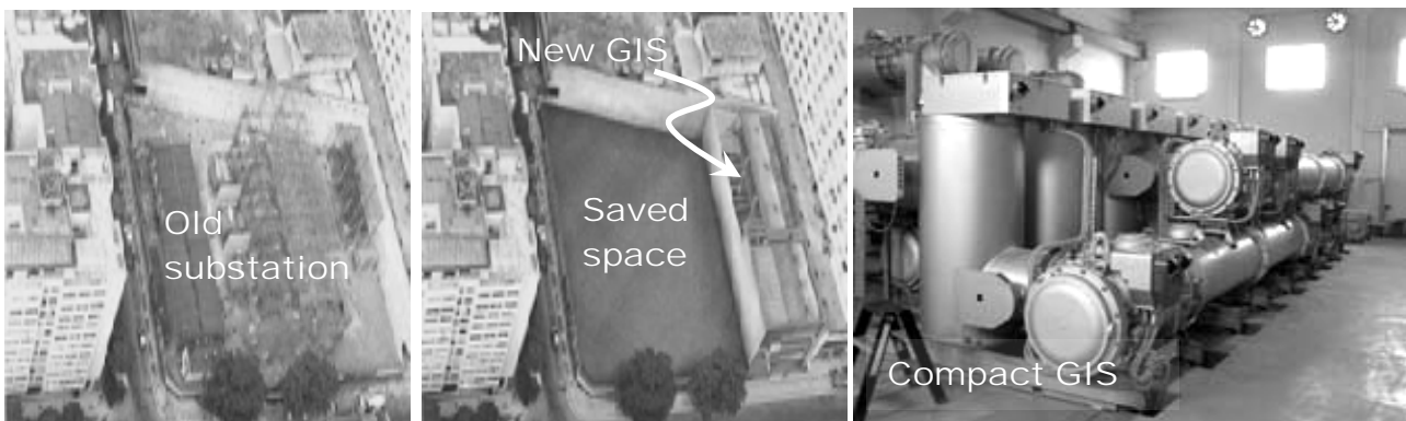
Figure 5.4.20 Space-saving characteristic of gas insulating substations (GIS) makes these substations ideal for operation in urban residential environments.
