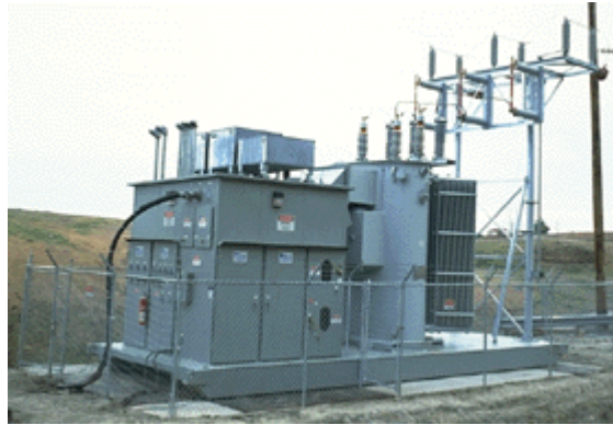
Figure 5.4.14 Substation in a rural area.
