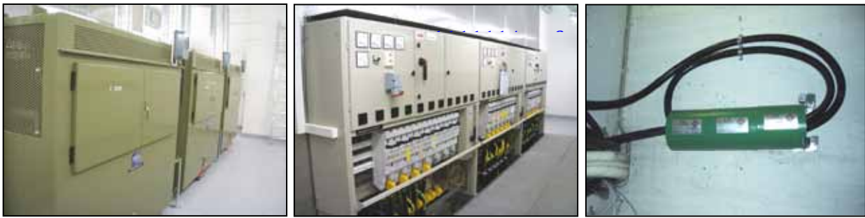
Figure 6.3.3 Some of the measures taken to mitigate the field from the substation under the City Library.
