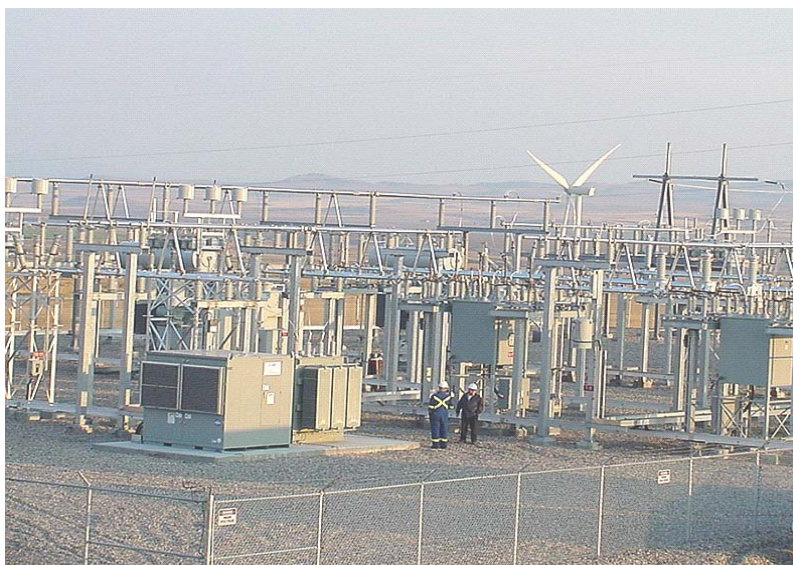
Figure 6-3 4MVAR D-VAR module installed at a wind farm substation
