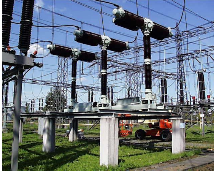
Figure 18 - Circuit-breaker B, three poles on a common structure
