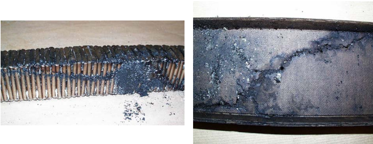
Figure 8 - Carbonisation and arc tracks along the stack (left) and in the supporting pressboard (right) of a partly short-circuited oil insulated grading capacitor
