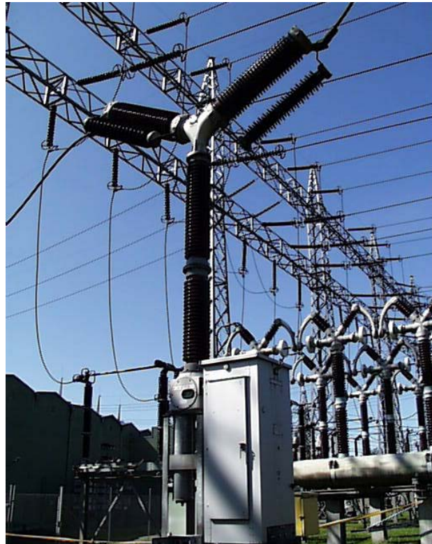
Figure 17 - One pole of circuit-breaker A
