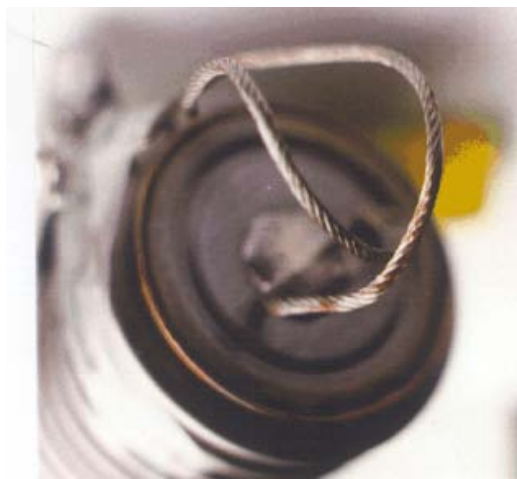
Figure 10 - Discolouration of the electric leads between bellows and end plate caused by discharge activity during disconnecter switching operations
