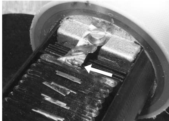
Figure 9 - Opened grading capacitor with partly broken foil conductor (see arrow).
