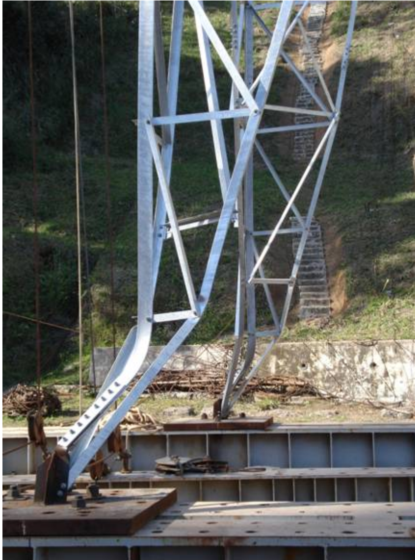
Figure 10.2 – Feet buckling during tests
