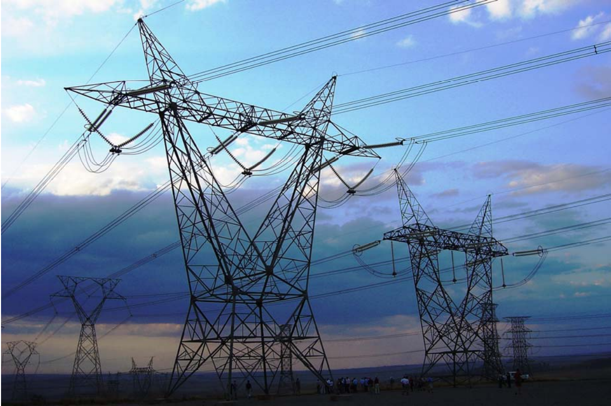
Figure 5 – 500 kV Transmission lines
