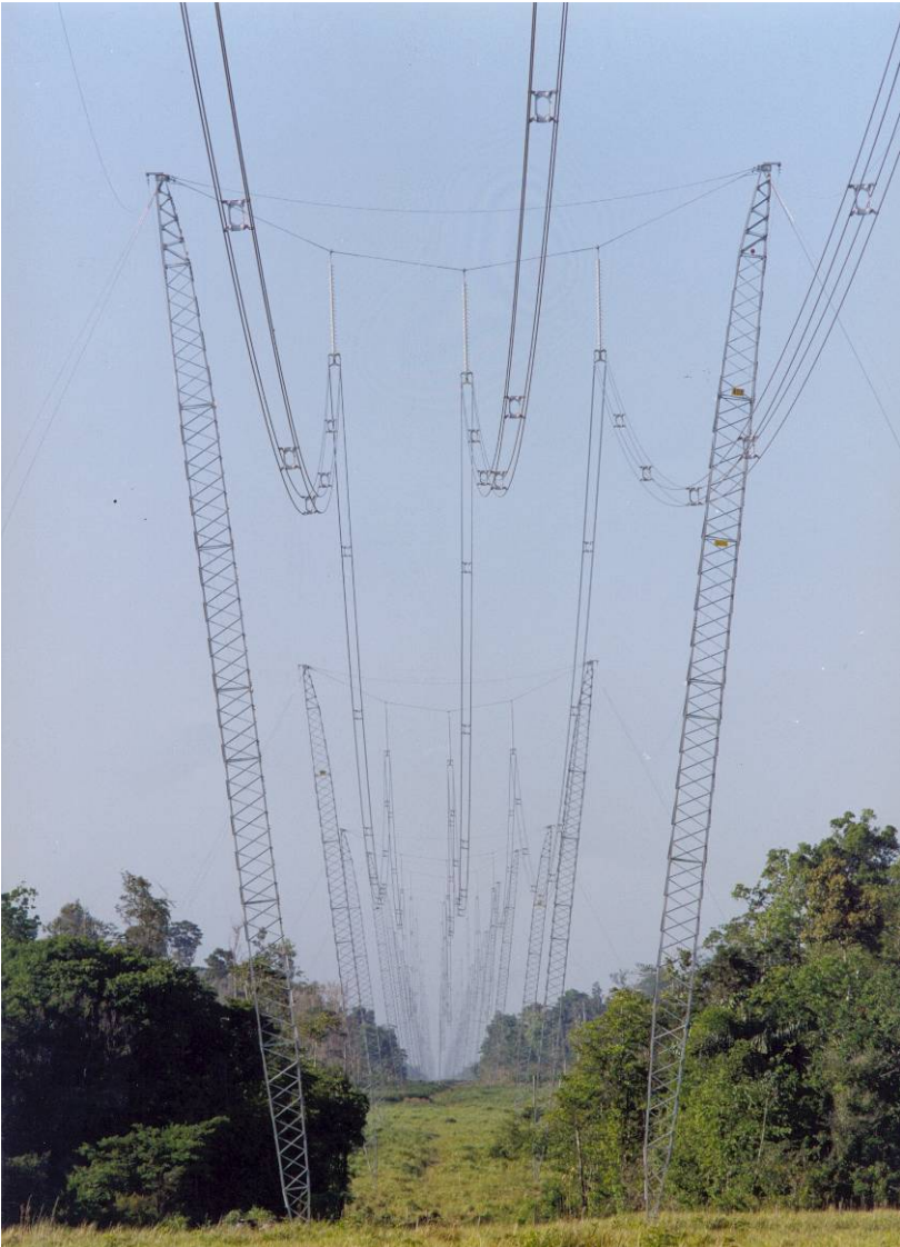
Figure 2 – 500 kV Cross Rope Suspension Tower
