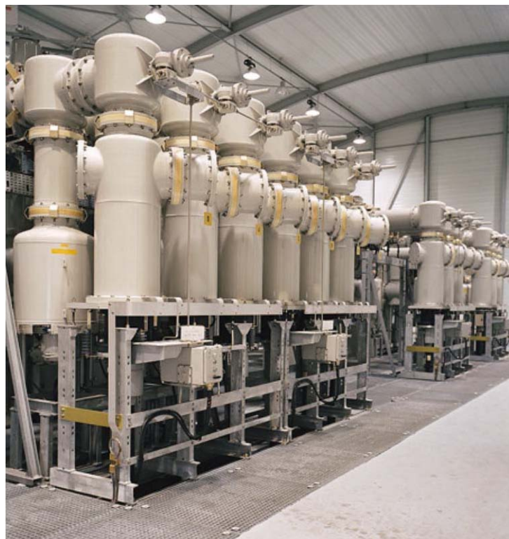
Figure 6: Gas Insulated Switchgear– © Médiathèque RTE / WEYL Laurent
