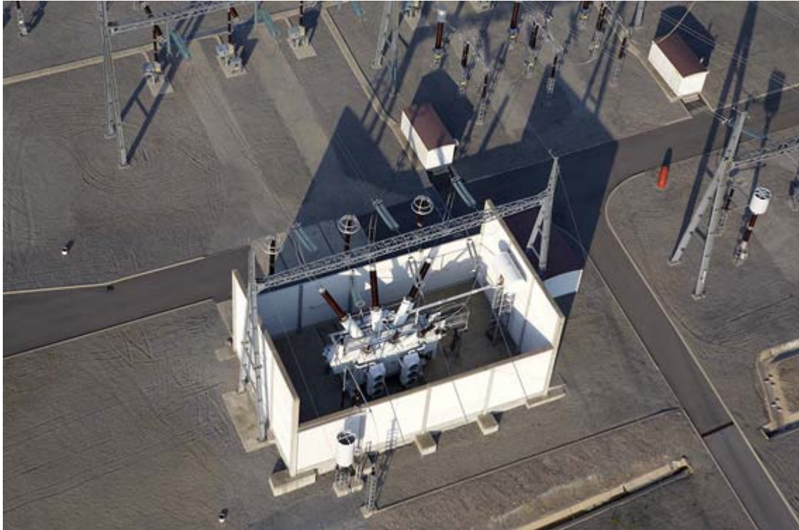
Figure 8: Transformer bay with fire walls and oil separator– © Médiathèque RTE / BARATIER Laurent
