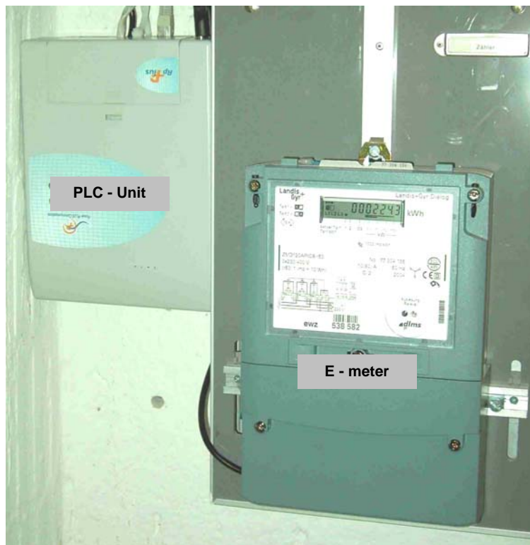
Figure 6-5 : Electricity meter installed with BB-Powerline
