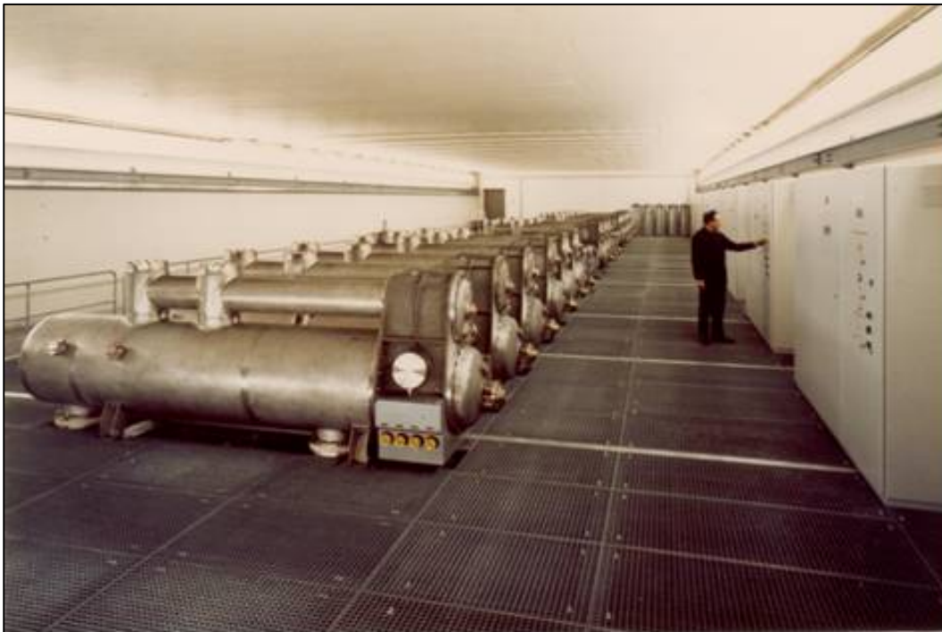
Figure 1.4 145kV GIS using SF6 Sempersteig Zurich 1968 (upper level)
