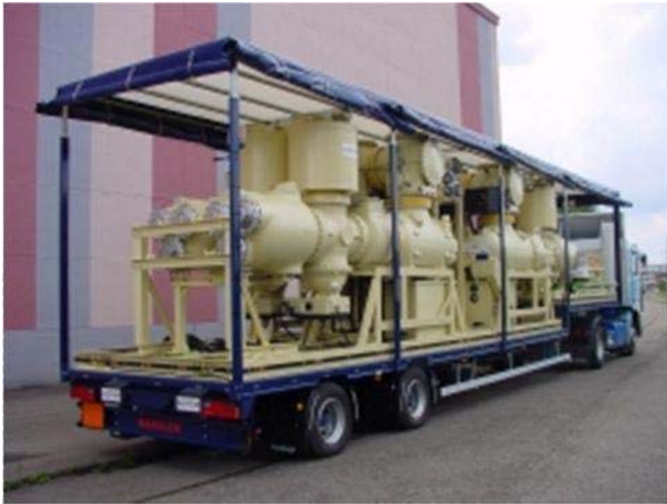
Figure 4.5.1 Mobile 145kV 40kA GIS Installation (4 bays)
