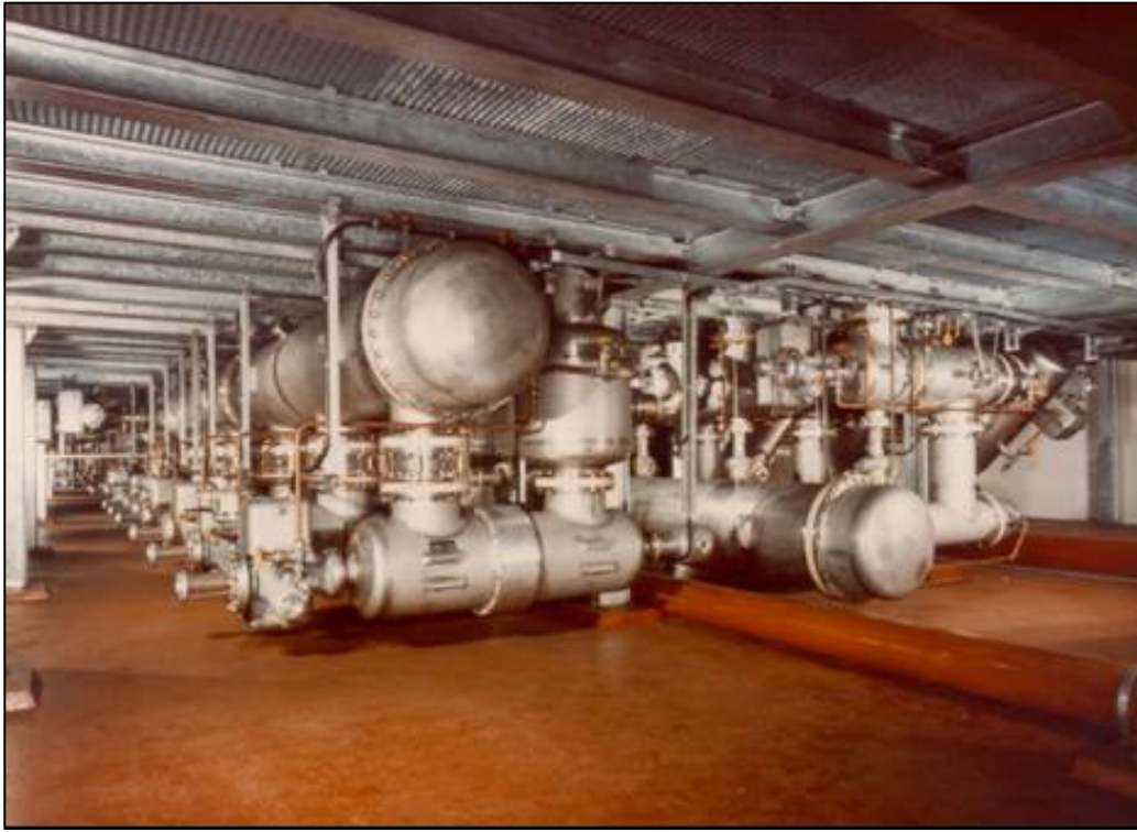
Figure 1.3 145kV GIS using SF6 Sempersteig Zurich 1968 (basement)
