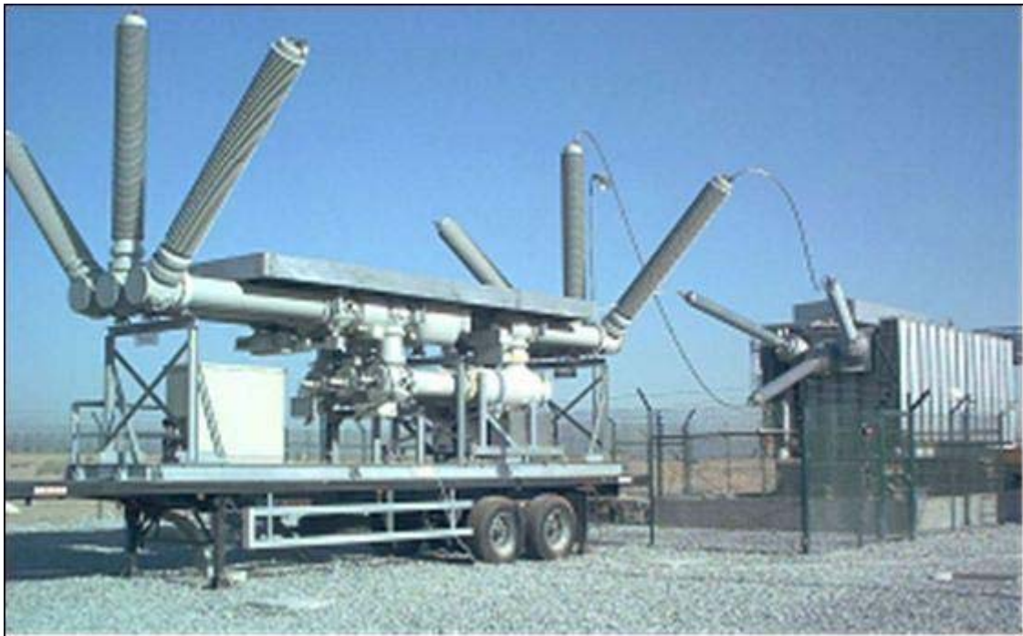
Figure 4.5.2 245kV 50kA Mobile Installation (1 bay)
