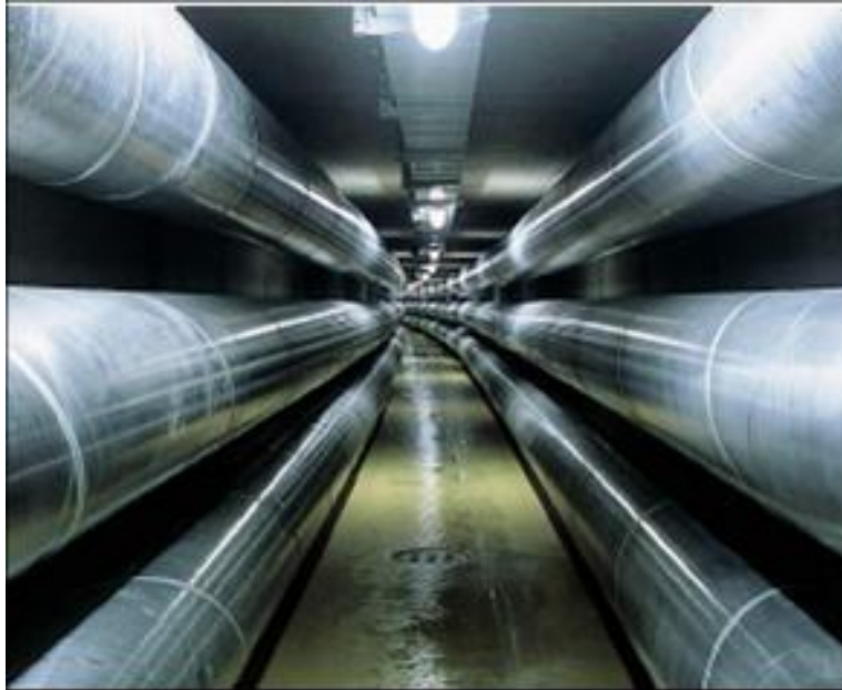
Figure 3.3.1 Gas Insulated Trunking in Tunnel
