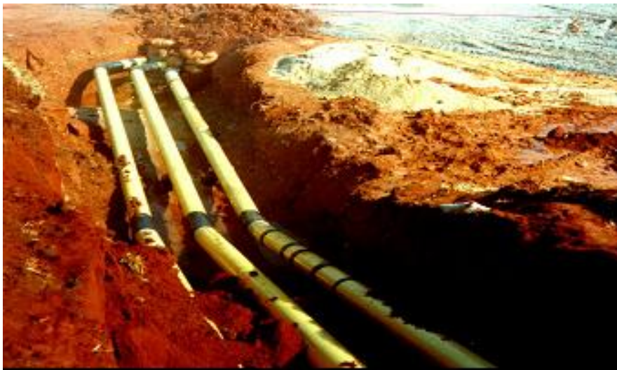
Figure 3.3.2 Gas Insulated Line - Direct buried.
