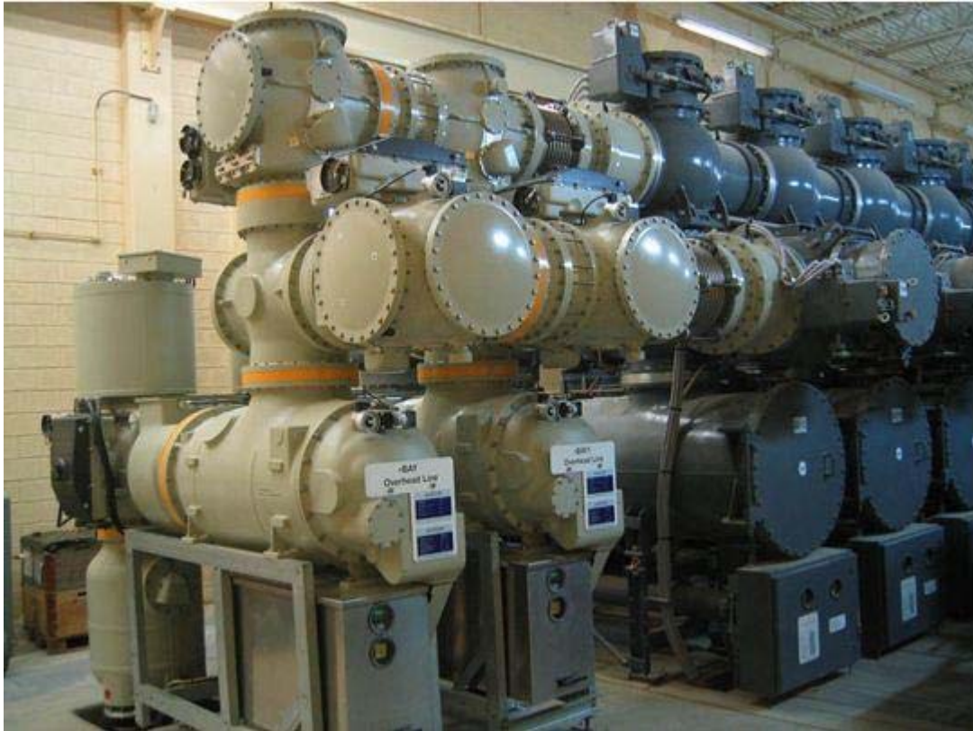
Figure 4.3.2 Extension of Existing GIS using new generation equipment from same original supplier
