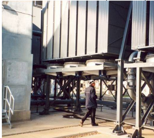
Figure 4 - QB large cooling outdoor fans (400 kV 2750 MVA)
