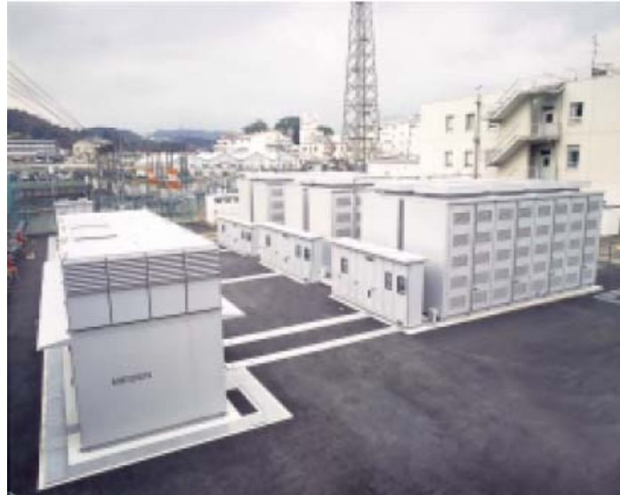
Fig 1. NaS 6MW battery storage system, Ohito substation Japan [1].
