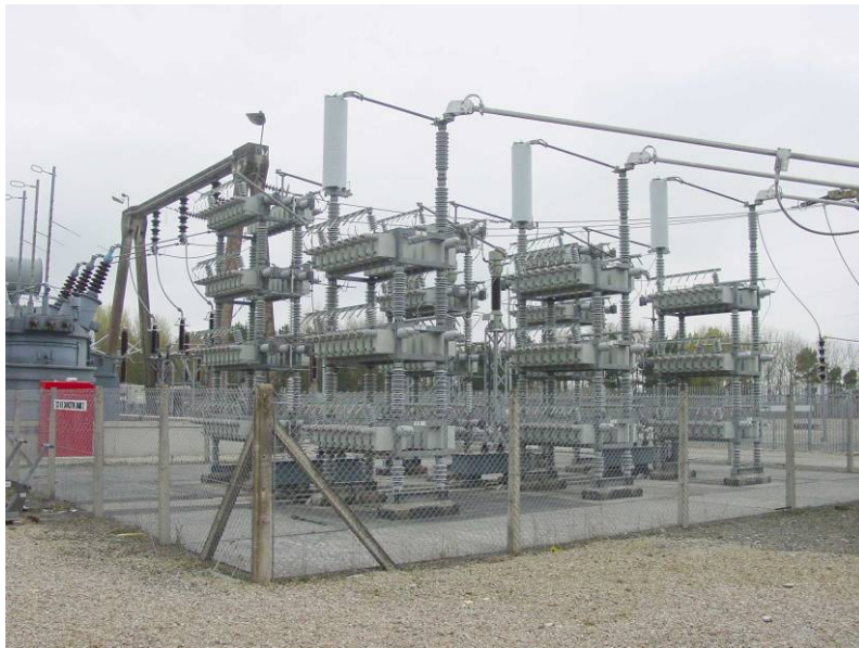
Fig 1. Typical 145kV capacitor bank
