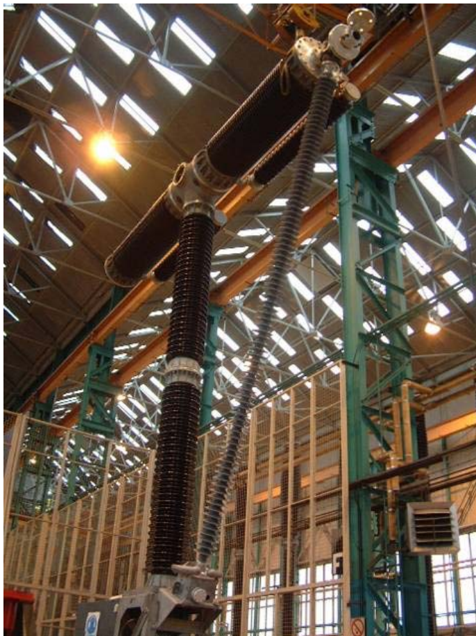
Fig 1. NCIT integrated with a circuit breaker [1]
