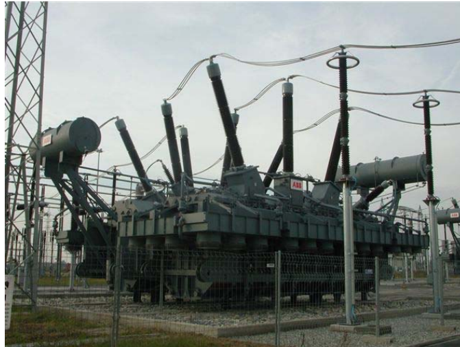
Figure 7. Outdoor 400kV QB 1650 MVA (Terna - Rondissone Substation)
