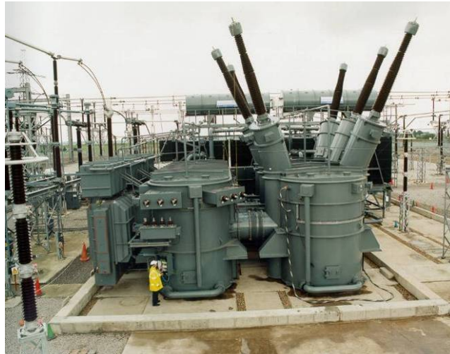
Figure 3 - 400 kV QB 2750 MVA
