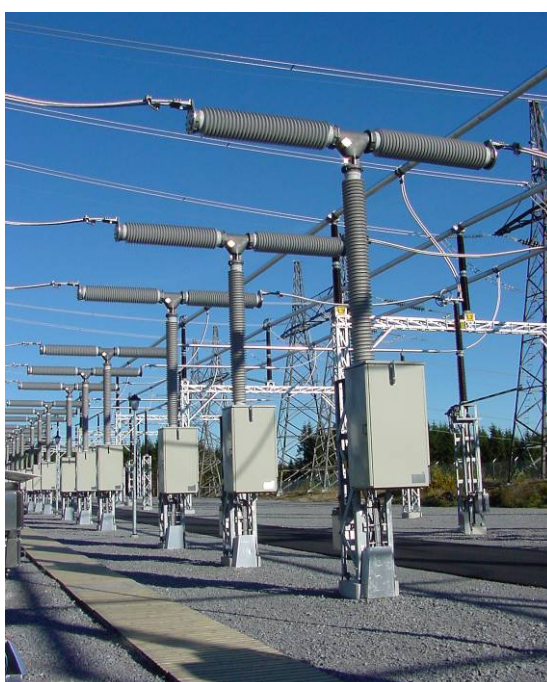
Fig. 2 420kV disconnecting circuit breaker
