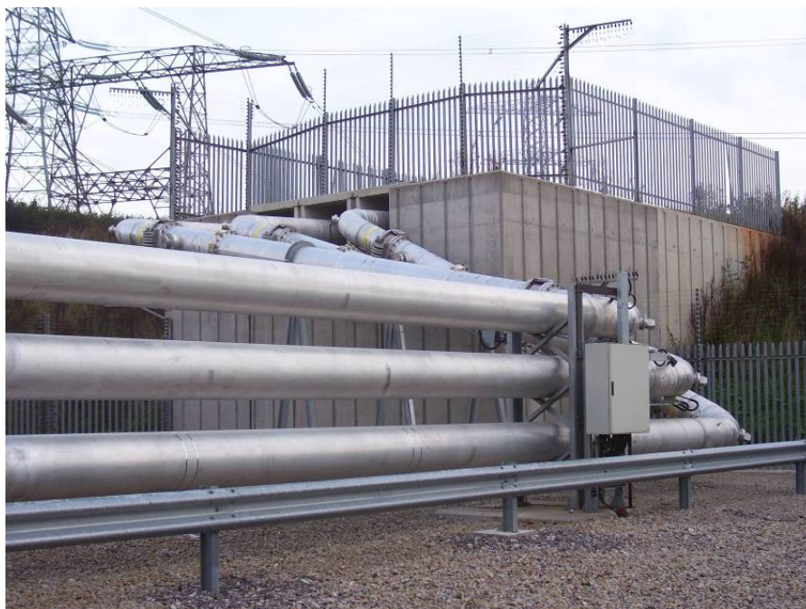
Fig 1. Gas Insulated Line [2]
