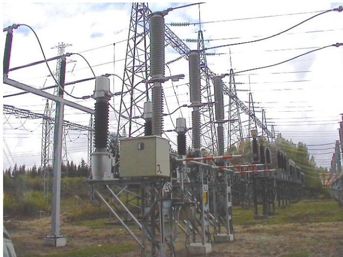
Fig 1. 145kV disconnecting circuit breaker
