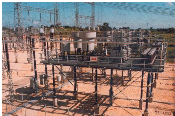
Figure 11 - TCSC - 500 kV (Brazil – Imperatriz substation)
