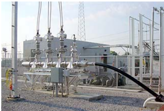
Fig 1. Example of a super conducting cable sealing end – AEP Bixby substation, USA.
