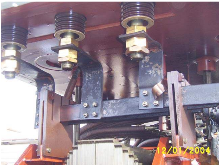
Fig 1h Formation of copper sulphide on leads in 20/30kV industrial transformer. from [4]
