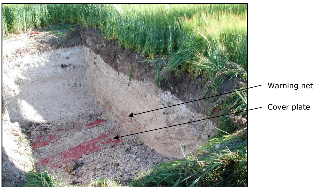
Figure 4.11 Cover plate on top of cables. The warning net can be seen on the right-hand side over the cover plate
