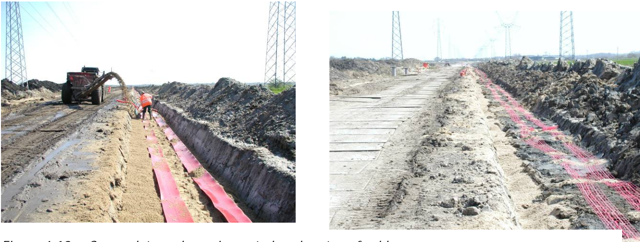
Figure 4.10 Cover plate and warning net placed on top of cables
