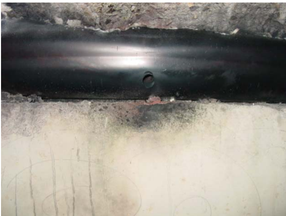
Figure 6.1 Cable damage caused by drilling
