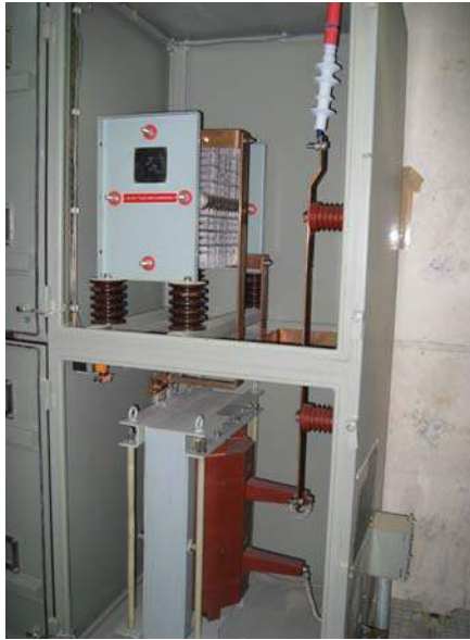
Turbogenerator: 312 MVA, 17kV, 50Hz Neutral grounding transformer: 12kV/240V, 25kVA, 50Hz, 10kA-1seg, 400A-1min. Secondary grounding resistor: 525 mOhm, 400 A-1 min.
