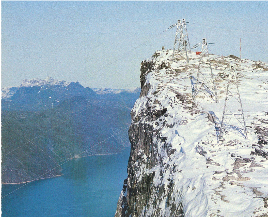
Figure 4: 132 kV Ameralik Fjord Crossing, Greenland
