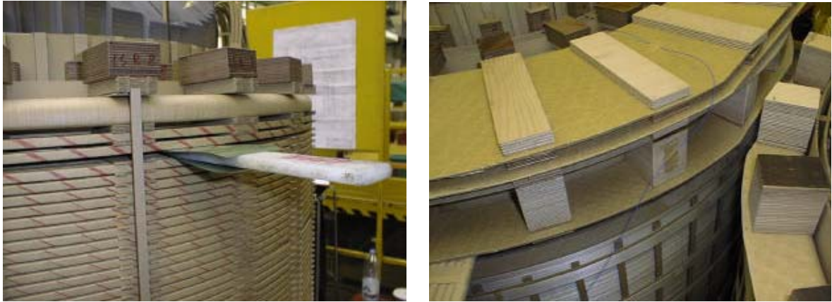
Figure 3-4: Left: Using a wedge and 2 layers of smooth material to replace a spacer. Right: Guiding the fibres to the top of the winding.
