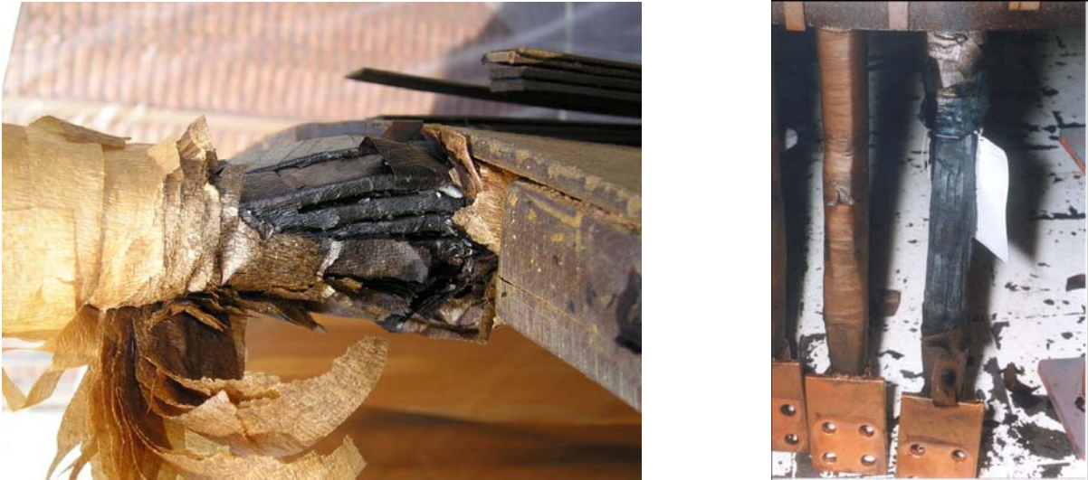
Figure 2-7: Predominantly pyrolytic destruction of overheated leads insulation.
