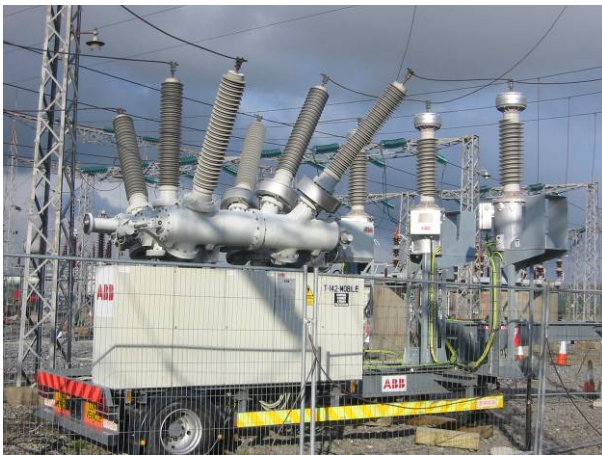
Fig. 3 110kV mobile bay
