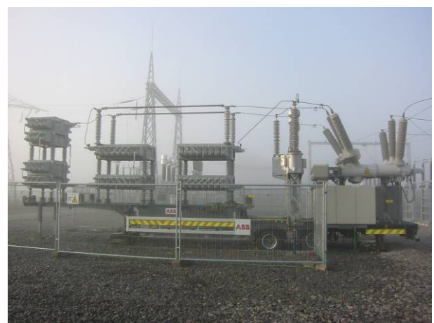
Fig. 4 Relocatable 110kV capacitor bank
