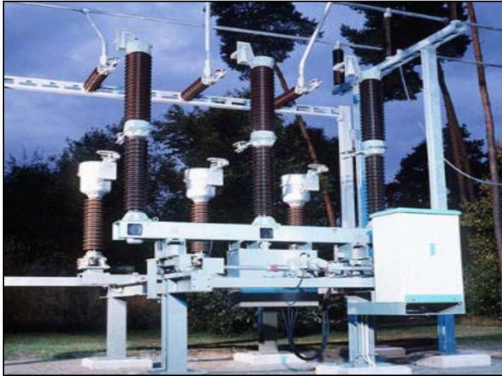
Fig 4: part of compact AIS Bay
