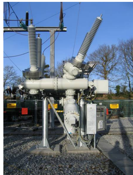
Fig. 8 MTS (AIS Busbar type)
