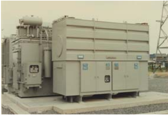
Old GIS Since 1980 (All in one cubicle type outdoor GIS / 100% Installation Space)
