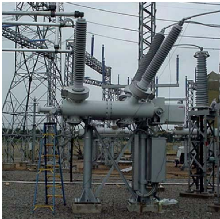
Fig. 3.1 Example – Hybrid modules used in a single busbar substation
