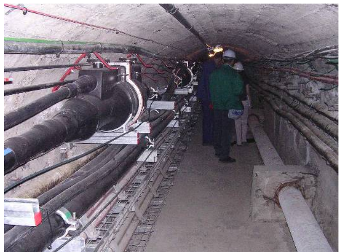
Figure 8.2.4 High Voltage power cable and joint in Madrid tunnel. Water main on floor opposite. (Courtesy of Iberdrola Ingeniería y Construcciones and Unión Fenosa)
