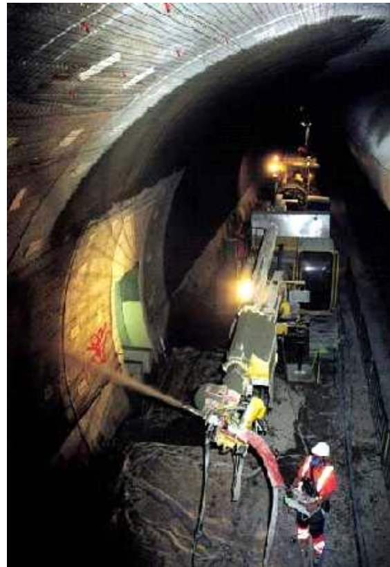
Figure 2.1.8 Fire protection sheathing of the inner lining of a tunnel (designed to withstand 1350° C)
