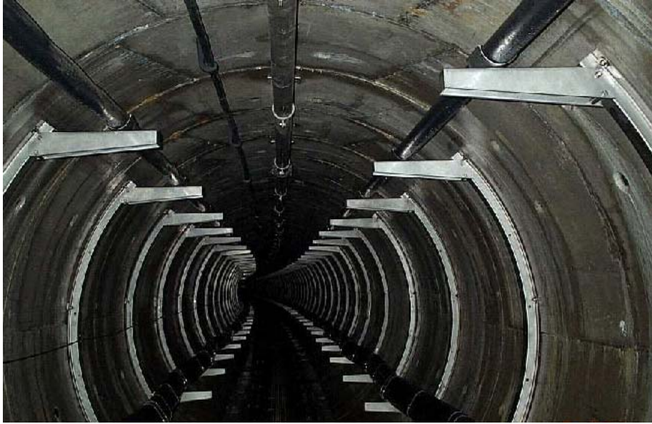
Figure 8.5.6 A general view of the Auckland Tunnel. Leaky co-axial communications cable and sprinkler system pipe installed on the ceiling. A drain is installed along the floor.
