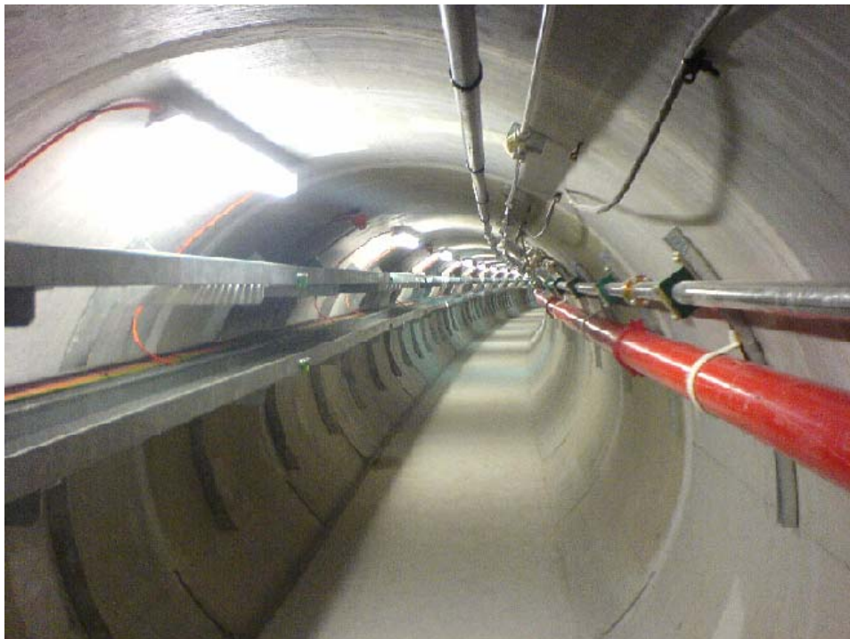
Figure 2.1.6 A completed pipe jack cable tunnel suitable for four circuits of high voltage cables
