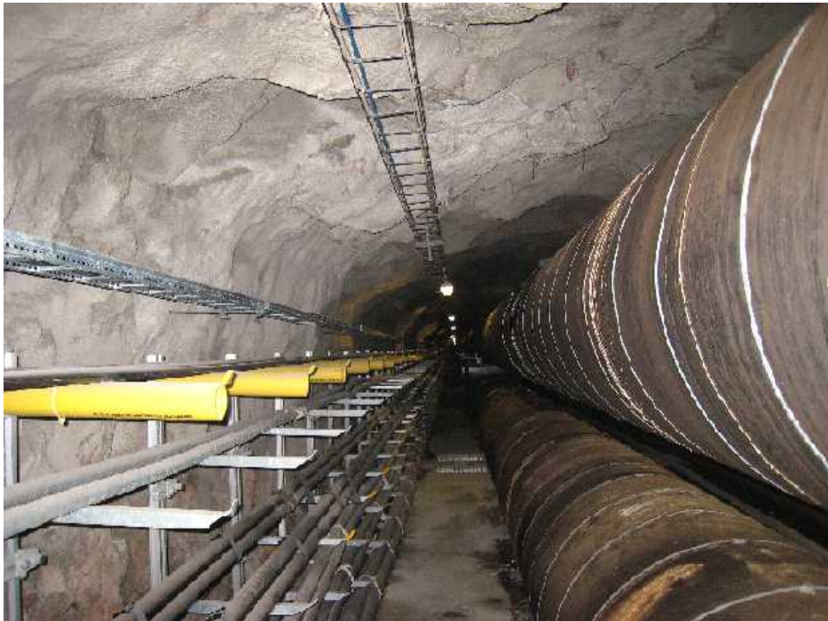
Figure 8.6.1 Typical Multipurpose Tunnel in Stockholm (shared with water pipes and communications)
