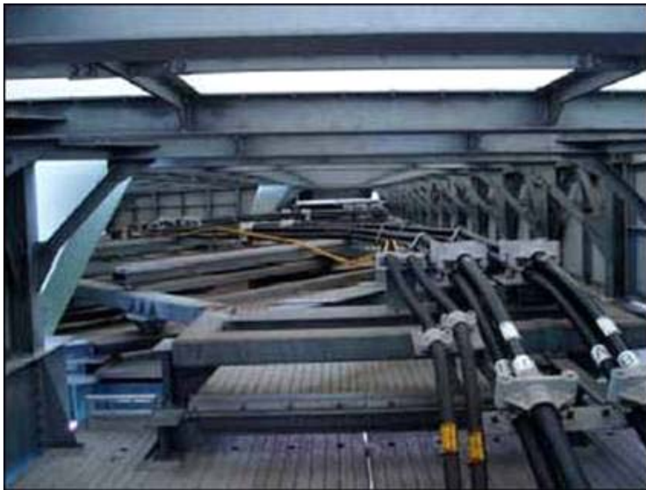
Figure 2.2.2 HV XLPE cables installed in a giant pantograph on a long suspension bridge
