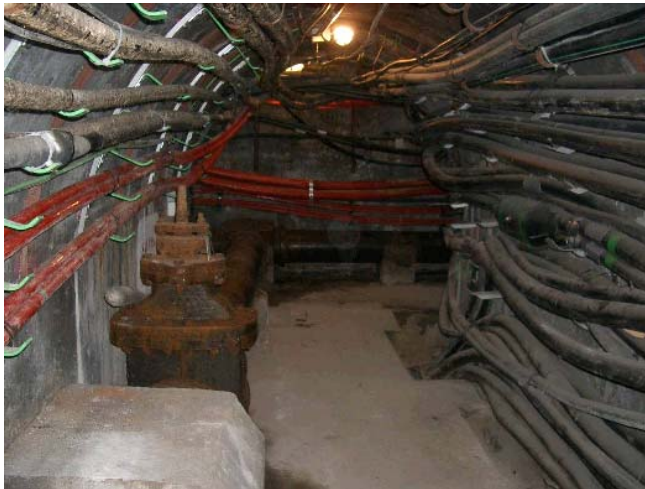
Figure 8.2.5 Water main (with valve) and power cables in Madrid tunnel. (Courtesy of Iberdrola Ingeniería y Construcciones and Union Fenosa)
