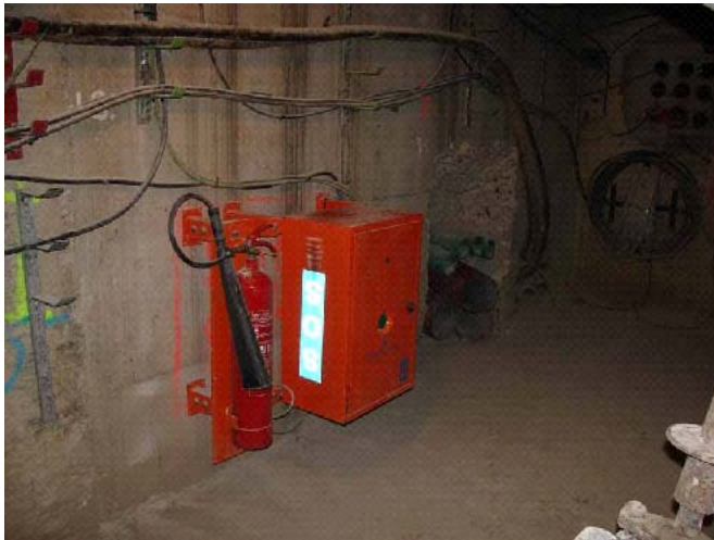
Figure 8.2.3 A SOS box in Madrid tunnel. Also pipes extended into the tunnel. (Courtesy of Iberdrola Ingeniería y Construcciones and Unión Fenosa)
