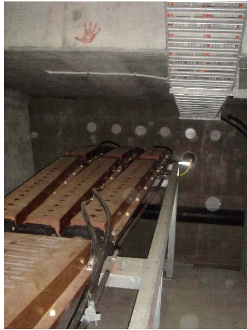
Figure 8.5.5 EMF shielding at exit points from the bridge where cables are no longer in trefoil
