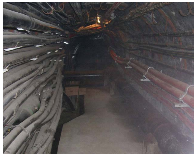
Figure 8.2.6 Section of a Madrid tunnel showing a water main at floor level with power and communication cables on the walls. (Courtesy of Iberdrola Ingeniería y Construcciones and Union Fenosa)
