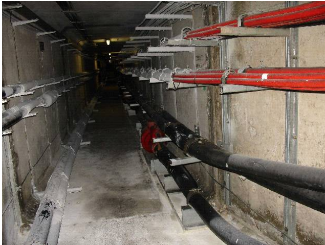
Figure 8.2.7 220 k V H V Cables ( with joints) on w all brackets in a Barc elona tun nel. Th e r ed conduits above left are for optical fibre communications. (Courtesy of Fecsa-Endesa)
