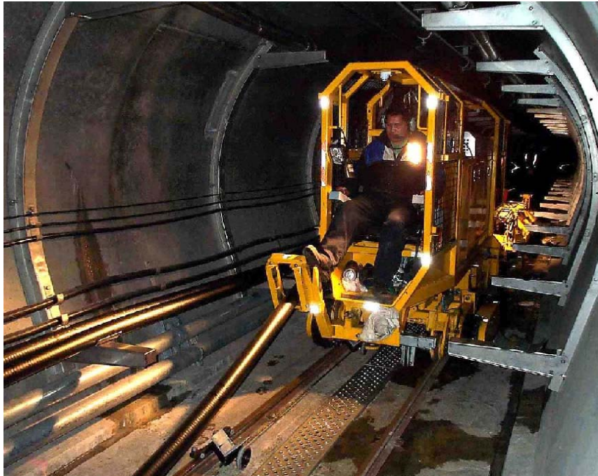
Figure 8.5.8 A special machine on guide rails was used to mount cables on wall bracketed cable cleats
