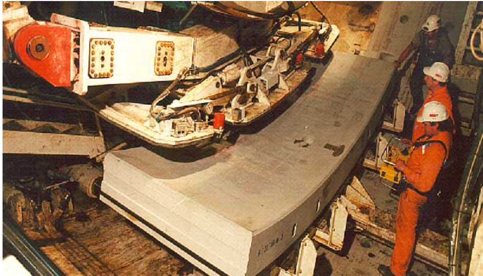
Figure. 2.1.5 A pre-cast segment is made ready to be hoisted into position within the tunnel
