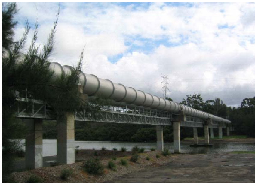
Figure 8.5.1 A 330 kV cable circuit installed in a mesh enclosure between water mains on a shared river crossing
