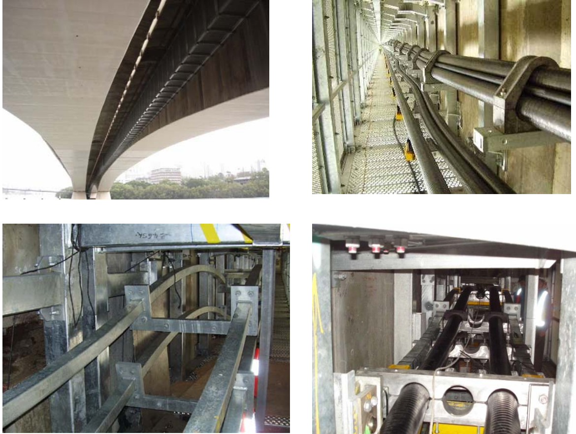
Figure 8.5.2 The steel structure for the cables that was retrofitted to the underside of the bridge and examples of the complex bow structure to prevent damage to the cables from bridge movement
