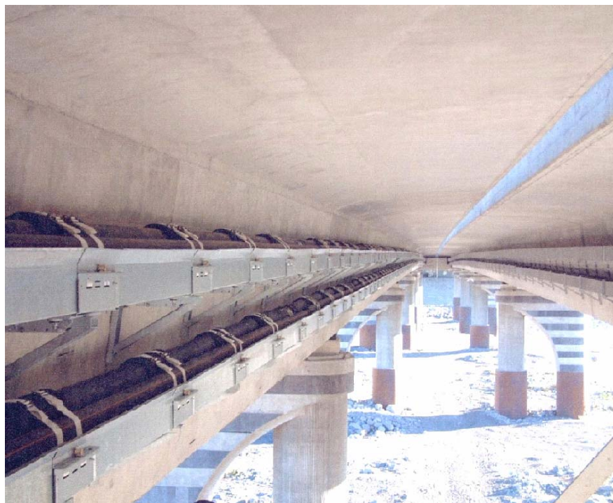
Figure 8.8.1 An example of cables installed in troughing under a bridge in France
