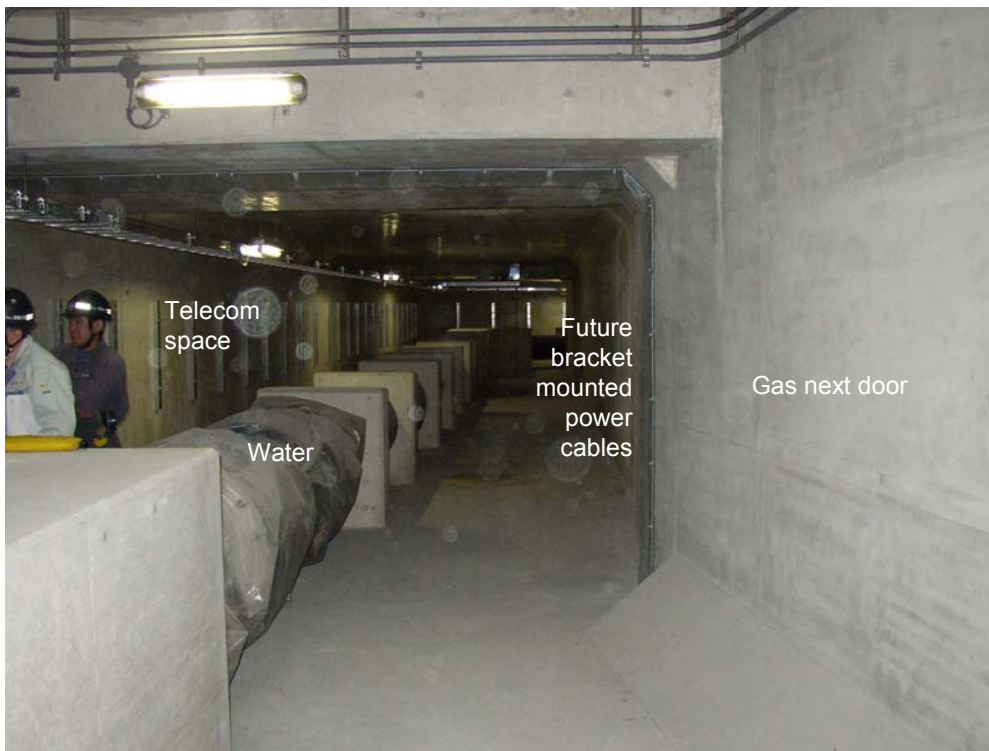
Figure 8.3.5 Example of a Multi Purpose Tunnel with the gas main in a separate compartment in the tunnel
