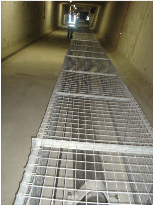
Figure 8.5.4 Cables inside the bridge structure were horizontally snaked enclosed in mesh
