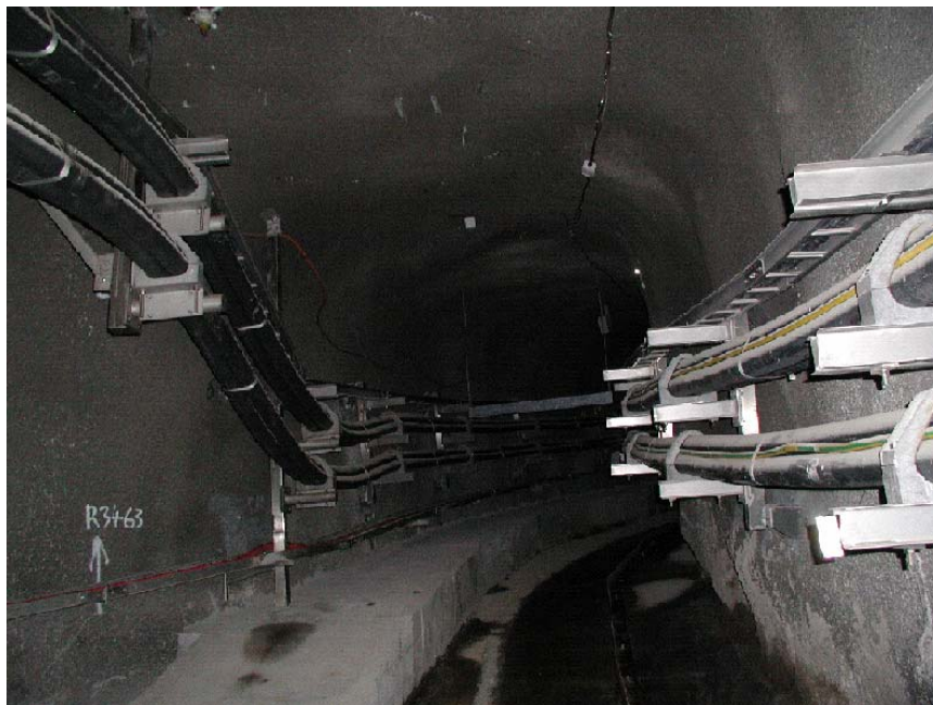
Figure 8.5.9 Tunnel shared by TCO and Distributor for HV Feeders in the Sydney CBD The bracket mounted 132kV cables are single point bonded.
