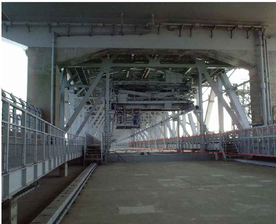
Figure 8.3.2 Location of the HV power cables on one of the suspension bridges (highlighted in red)
