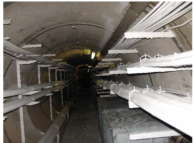
Figure 8.2.8 A section of Barcelona tunnel where HV cables are mounted below MV distribution and service cables are treated with a white flame retardant coating. (Courtesy of Fecsa-Endesa).
