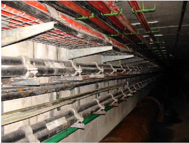
Figure 8.2.1 Power cables and communication cables in a Madrid tunnel (Courtesy of Iberdrola Ingeniería y Construcciones and Union Fenosa)
