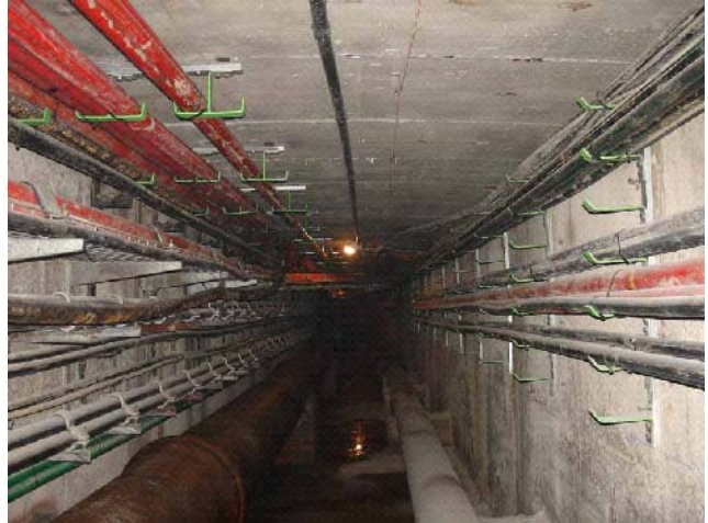
Figure 8.2.2 View of a Madrid tunnel showing water pipes on the tunnel floor. (Courtesy of Iberdrola Ingeniería y Construcciones and Unión Fenosa)
