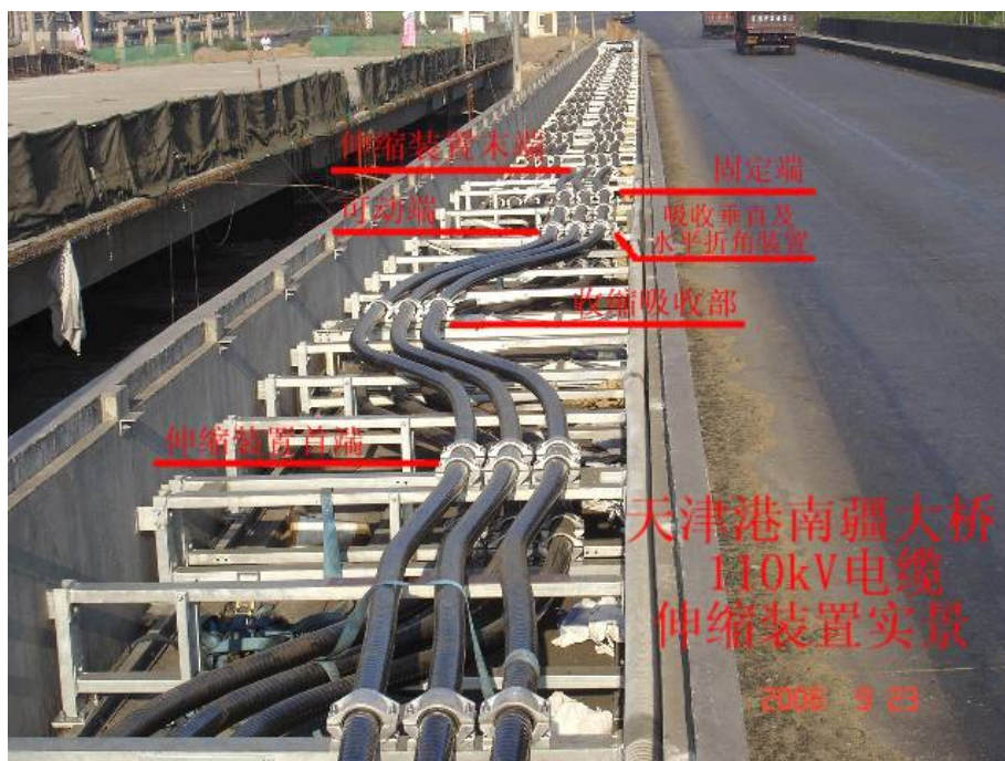
Figure 8.4.3 A typical snaking arrangement for cables to allow for movement on the Tianjin Nanjiang Bridge
