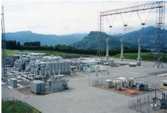
Fig. 105 UHV transformer under field test
