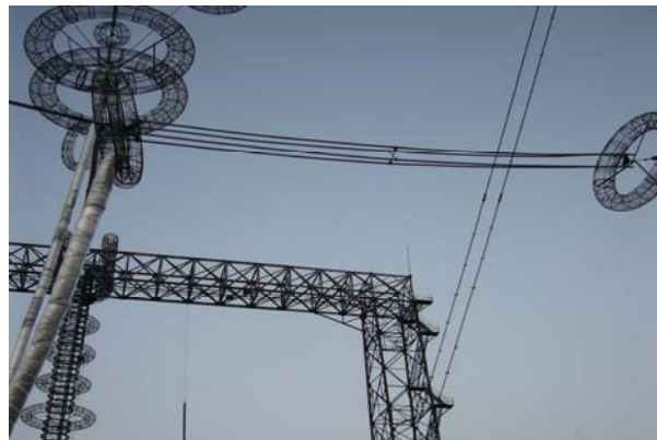
Fig. 23 Electromagnetic field test set-up for 4-bundle conductor
